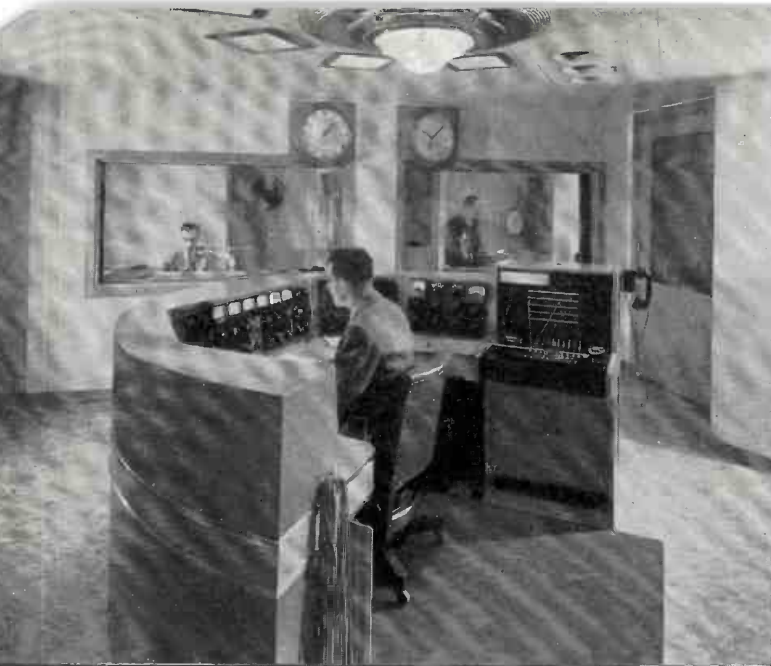
FIG. 1. (Top left) Master Control Room. From his position at the control desk, the engineer can view the operations going on in the eight studios which are grouped around the master control room.
