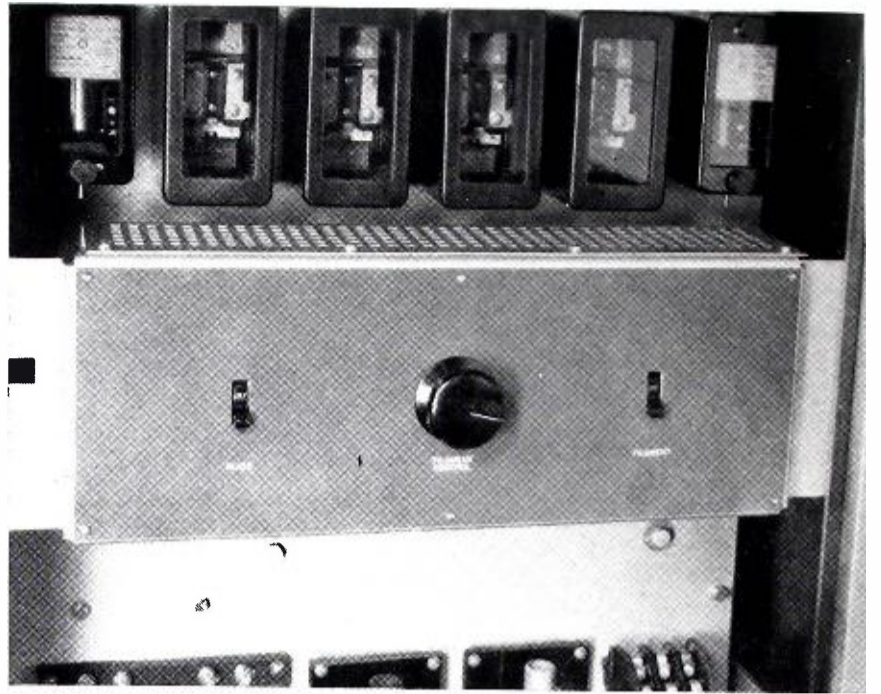
Circuit-breaker switches are located in all power circuits.
