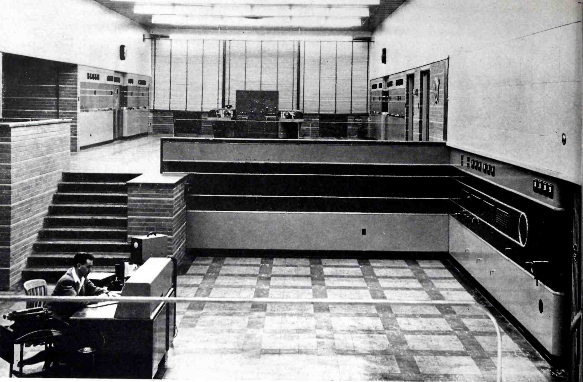
FIG. 3. On the mezzanine floor are two RCA 50-SW transmitters with monitoring, test and control equipment at center. On the lower floor is CBA'S standard band RCA Transmitter Type 50-D.
