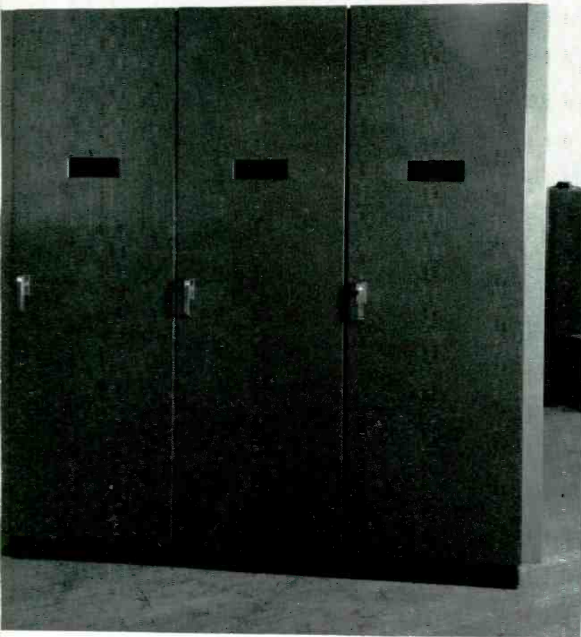
7. REAR of the unit-assembly shown on the preceding page. Full-length, full-width doors provide easy access. Peep-holes in door allow observation of equipment in operation.
