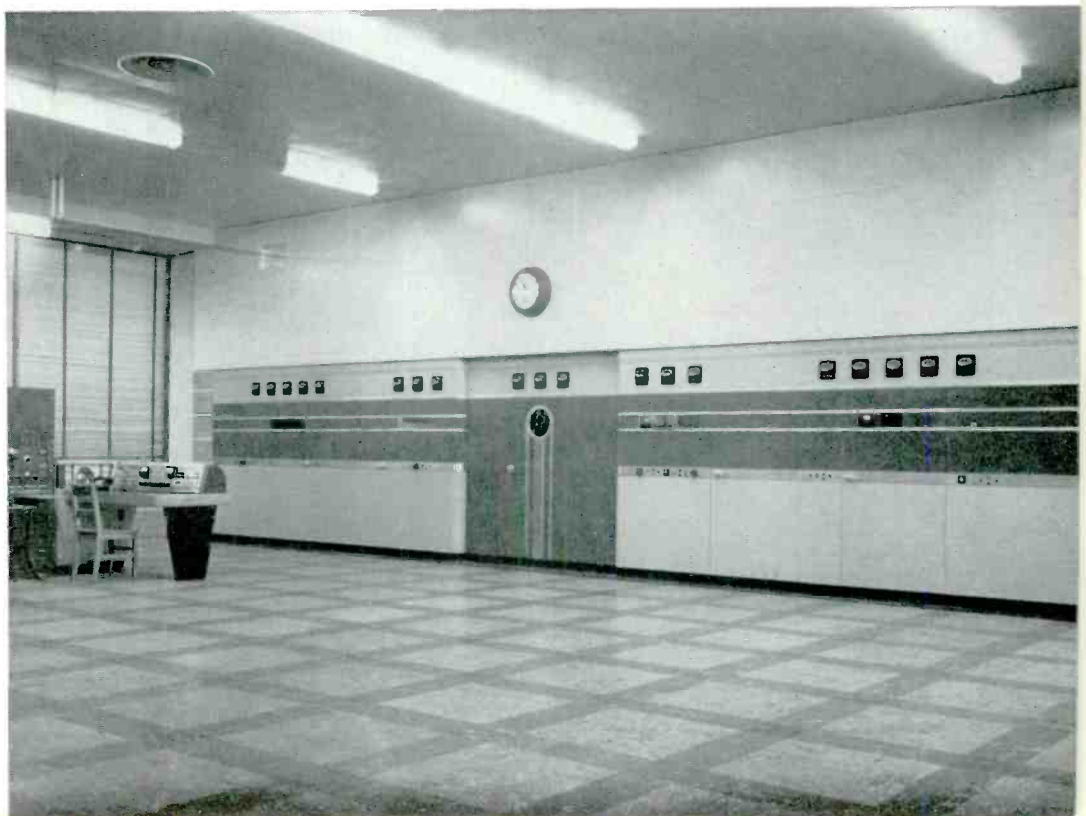
FIG. 6. Front view of RCA Type 50-SW #2 with control console and audio rack at left.
