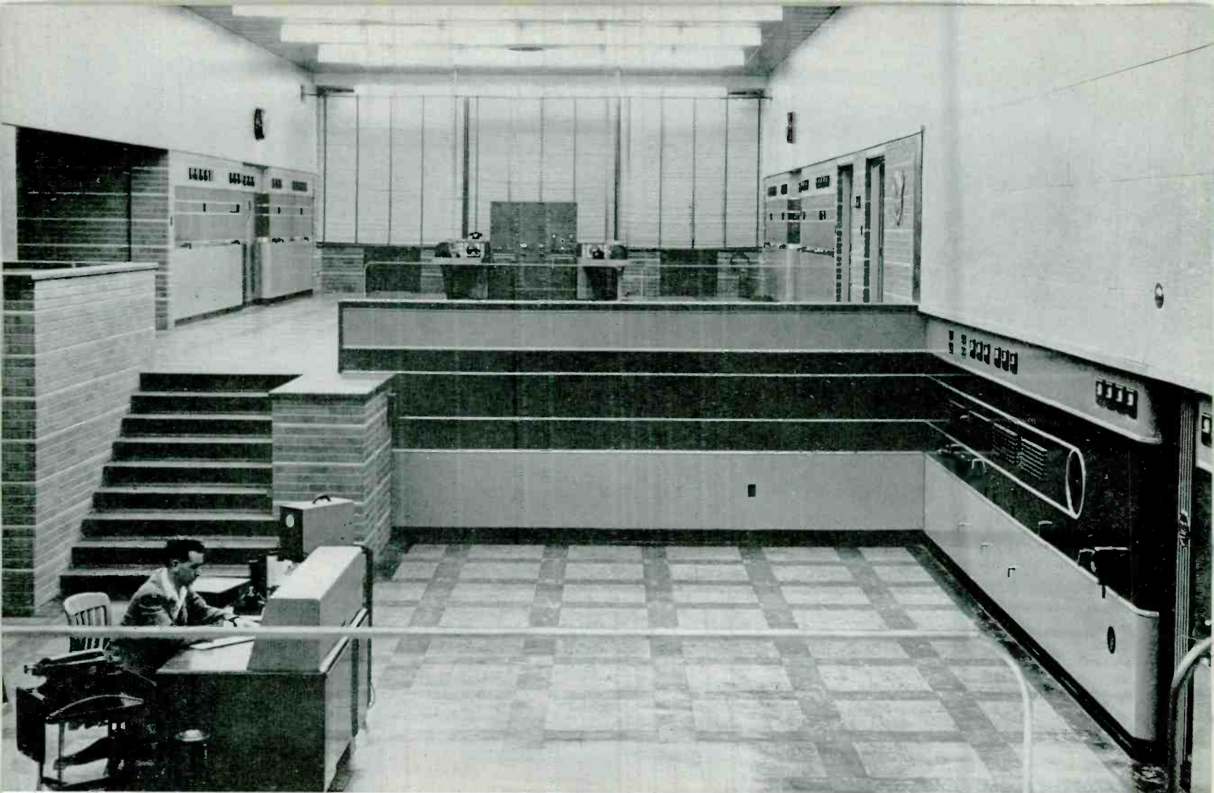
FIG. 3. On the mezzanine floor are two RCA 50-SW transmitters with monitoring, test and control equipment at center. On the lower floor is CBA'S standard band RCA Transmitter Type 50-D.
