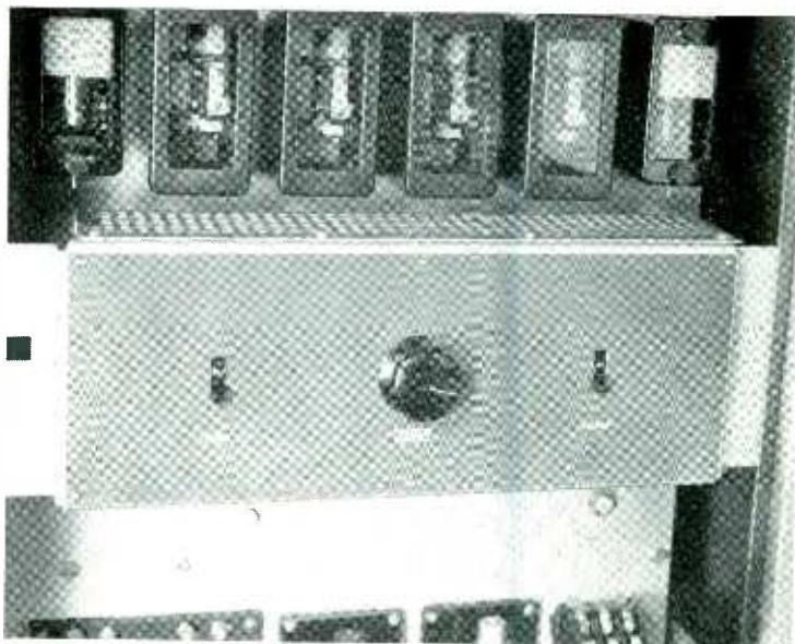
Circuit-breaker switches are located in all power circuits.
