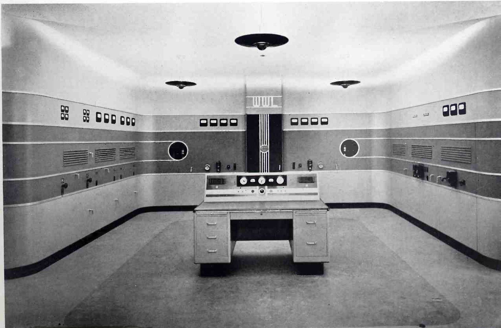
1938 WWL's fifty kilowatt RCA transmitter (shown below) was installed in a new building (see above) at a new site in 1938. It is one of the country's finest installations.
