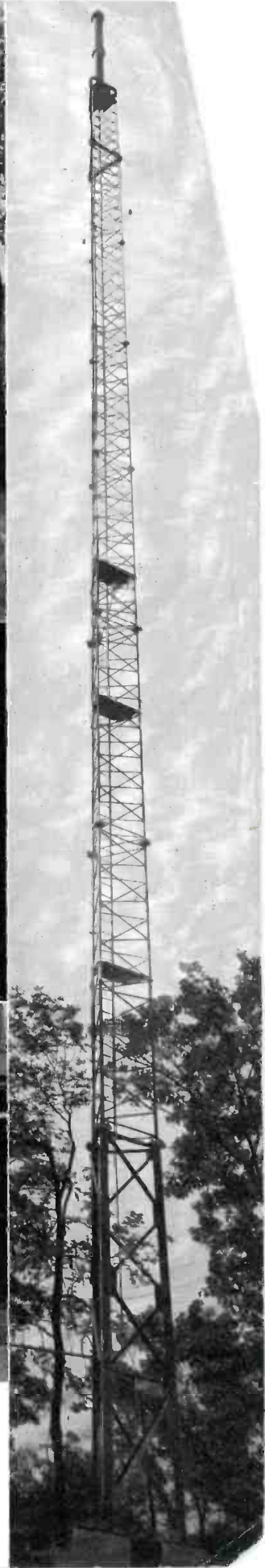
FIG. 5 (at far right). The WPAY-FM, two-section Pylon antenna mounted on a 173-foot tower. The RCA 3 KW FM transmitter and Pylon antenna provide an effective radiated power of 7,000 watts.
