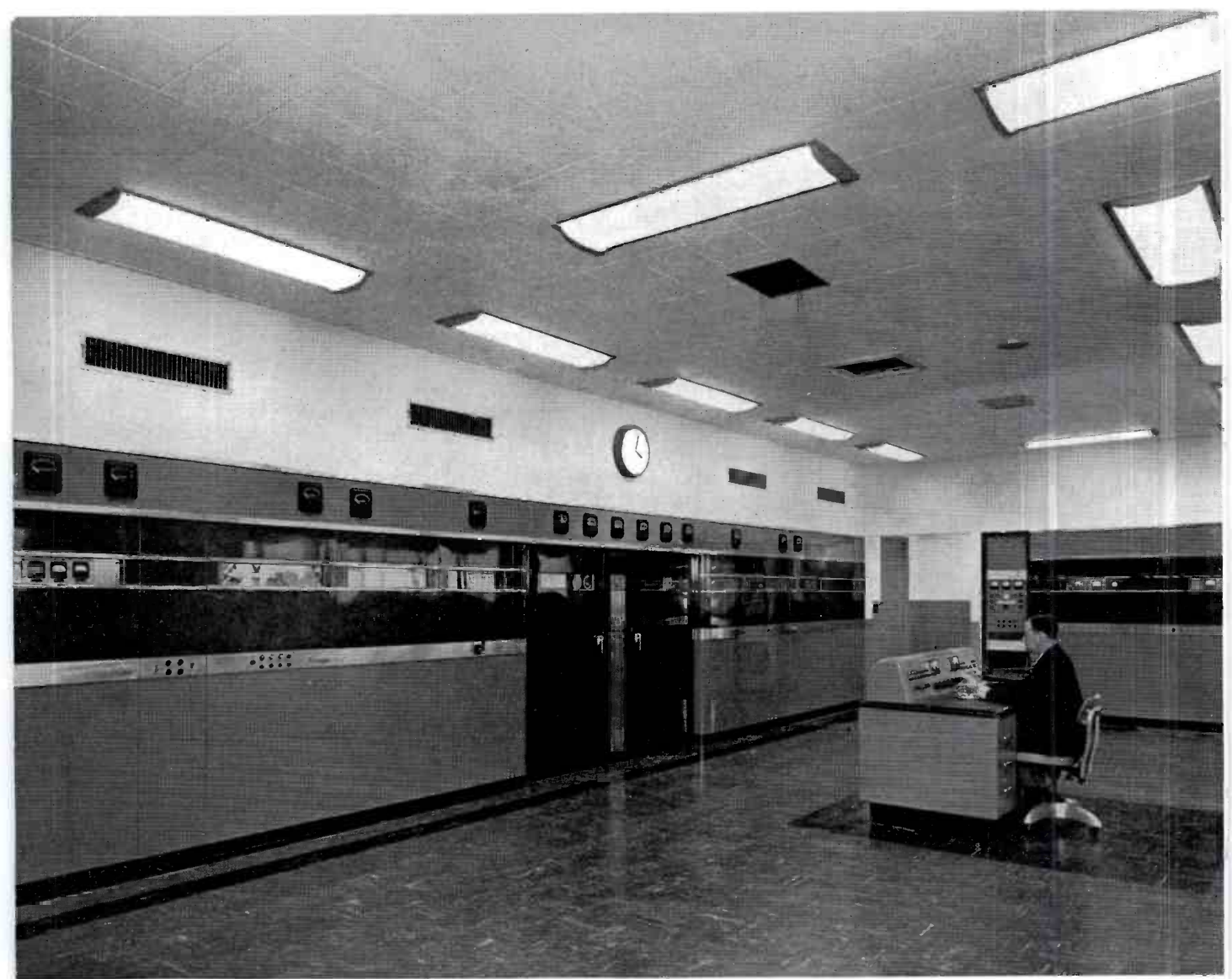
FIG. 2 (Above). The streamlined 50,000 Watt AM transmitter, Type RCA BTA-50F, is installed in the new transmitter building erected by KOMO on Vashon Island, approximately 20 miles from the broadcasting station in downtown Seattle. The supervisory control console contains extension controls for the transmitter as well as audio switching controls for regular operation.
