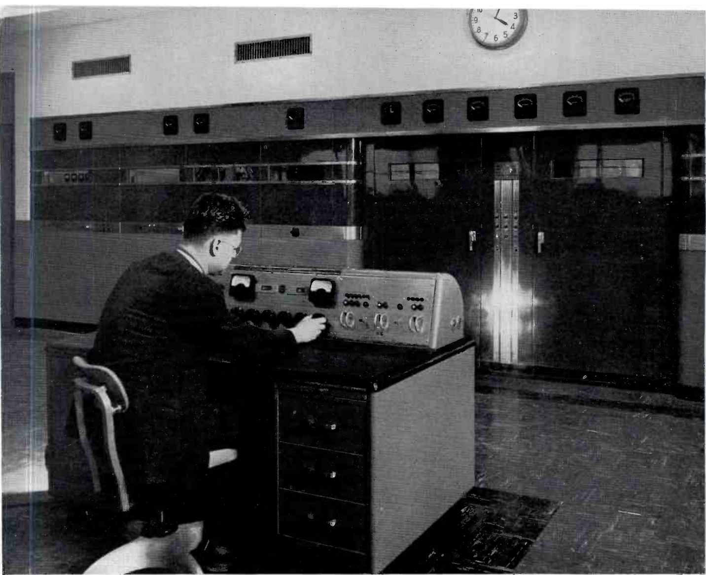
FIG. 3 (Above). KOMO's new RCA 50-F 50 KW transmitter and supervisory console. A concrete fireproof vault with automatic CO 2 equipment extends full length back of transmitter panels to house high voltage and modulation transformers.
