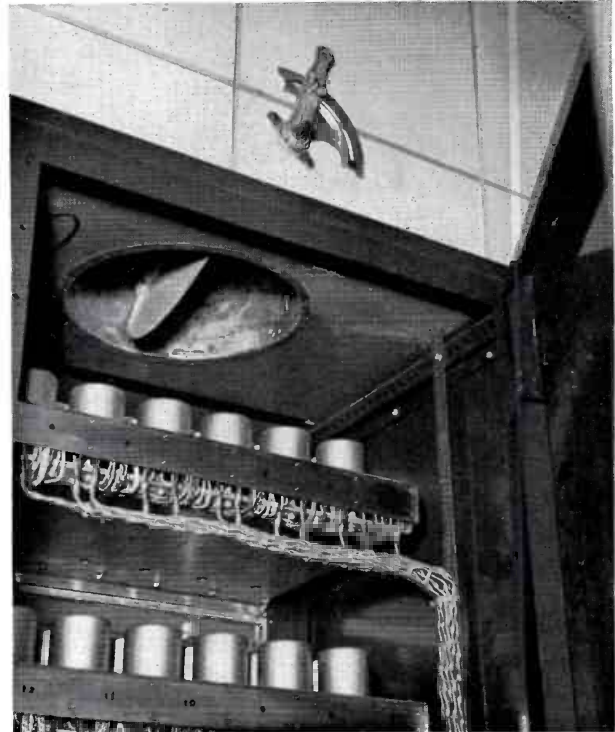
FIG. 13. A thermostat in the overhead duct controls the suction fans. Amount of air drawn from each of the racks can be controlled by dampers in the top of each rack, such as this one in the audio rack.
