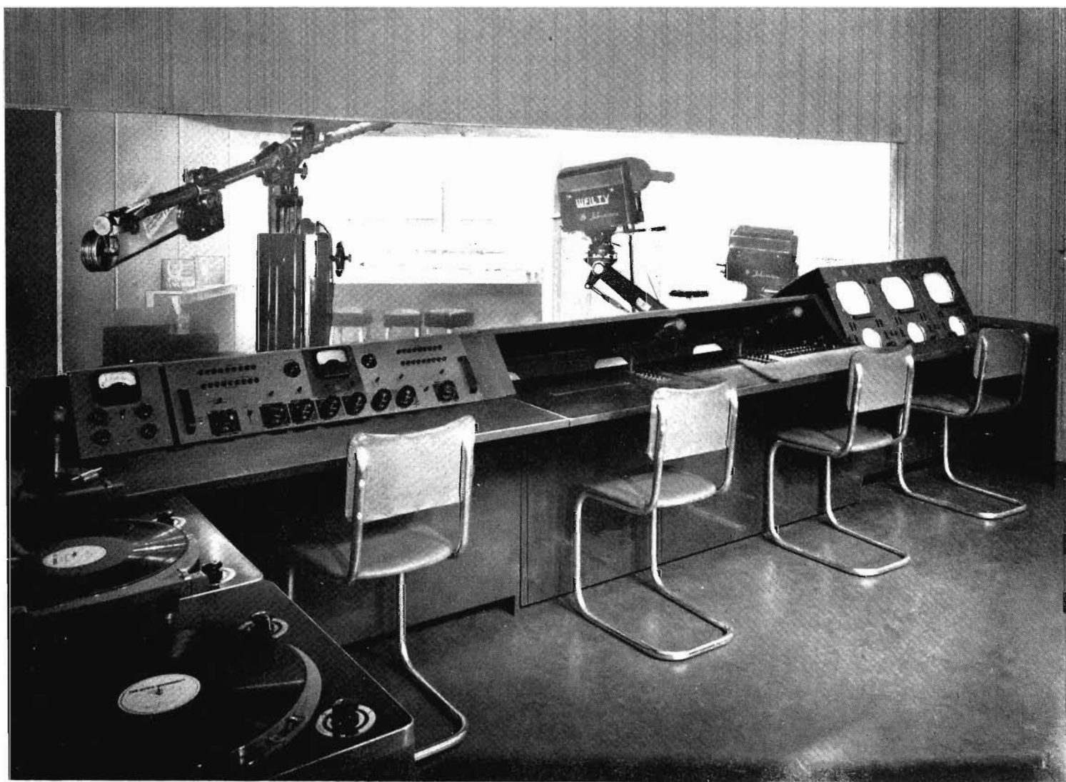
FIG. 32. One of the Studio Control Rooms in the Type F Station. This type station employs two or more studios each with similarly equipped control rooms. Several other physical arrangements of the unit-built control equipment are possible.
