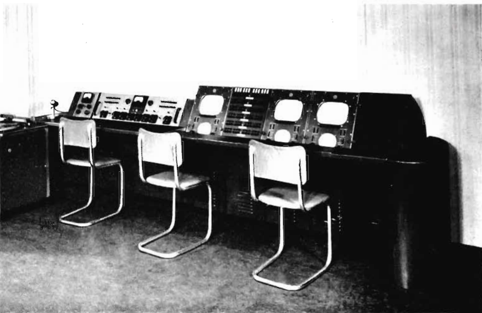
FIG. 33. The Type F "master" station employs separate control rooms for its studios, projection rooms and for master control functions. Above photo shows the master control console; below is the film control console. Diagram at right is a partial floor plan of the station.
