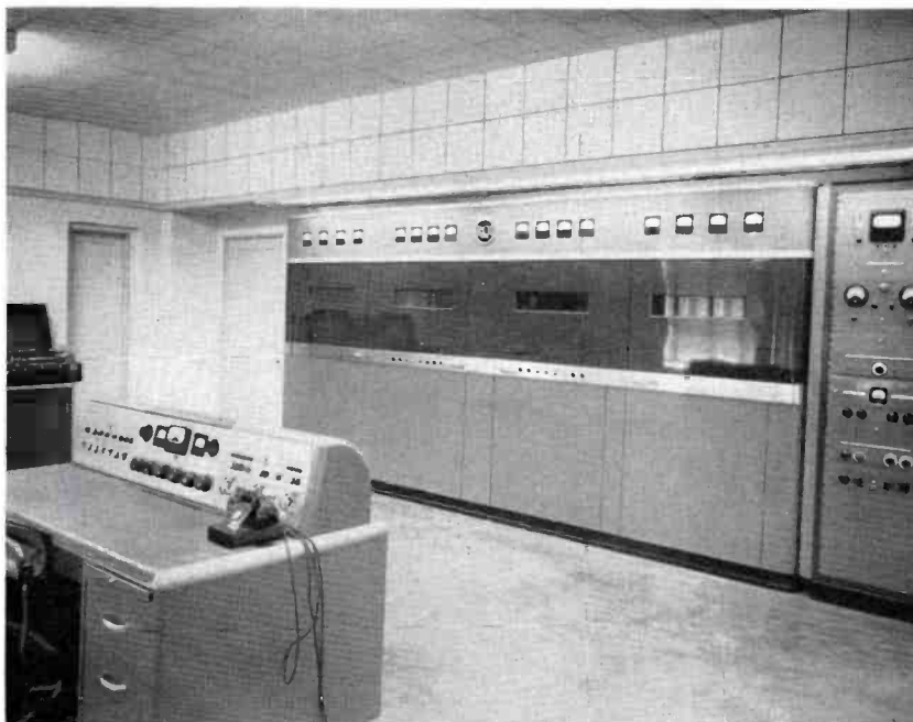
FIG. 1. Photo above shows the transmitter control room of Station KSEI. Recessed fluorescent lighting is used to illuminate the meters of the RCA 5 KW AM transmitter and the speech input racks. The transmitter control console is shown at left.
