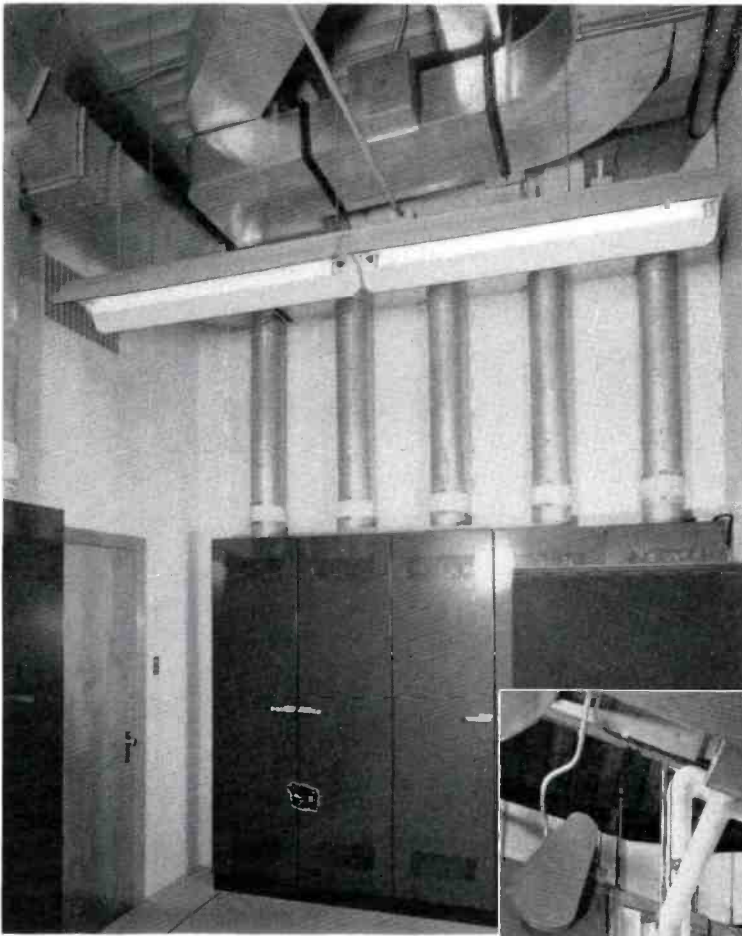
FIG. 16 (left). This is a view in the "test and storage" room adjacent to the studio control room. The back of the video cabinet racks (which face into the control room) is seen here. Ducts are used to exhaust heat from the equipment racks directly to the outside during the summer time, or for recirculating it to the station's heating system in cold weather.
