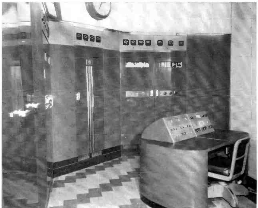
FIG. 12. The model of neat, flush construction is shown in this photo of WMAR-FM transmitter room. Station uses 10 kw RCA FM transmitter which feeds a two-section Pylon Antenna.
