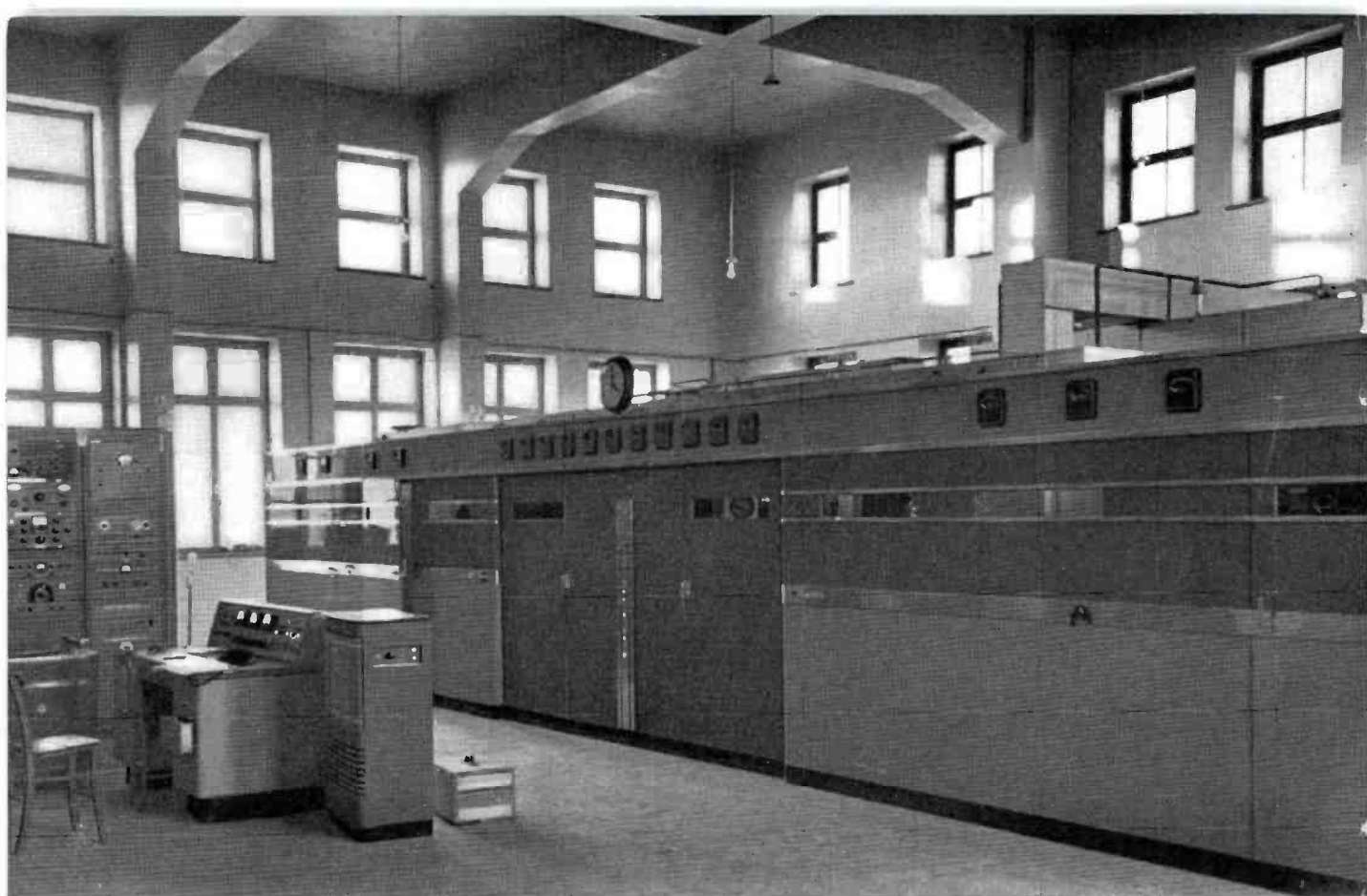
FIG. 1. The RCA Type BTA-150A Transmitter installed at Radio Istanbul, Turkey. The transmitter control console and test and measuring equipment racks are shown at left.
