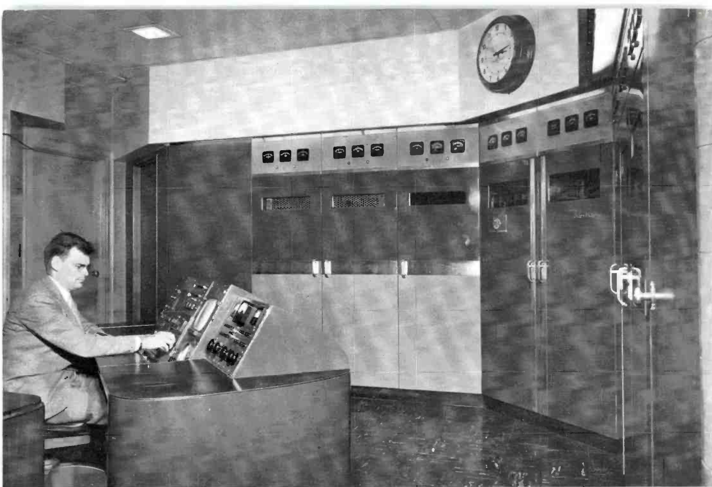
FIG. 10. C. B. Lau, Television Transmitter Supervisor, checks picture quality on TV transmitter control console. Note "U" arrangement of RCA TT-5A TV Transmitter.
