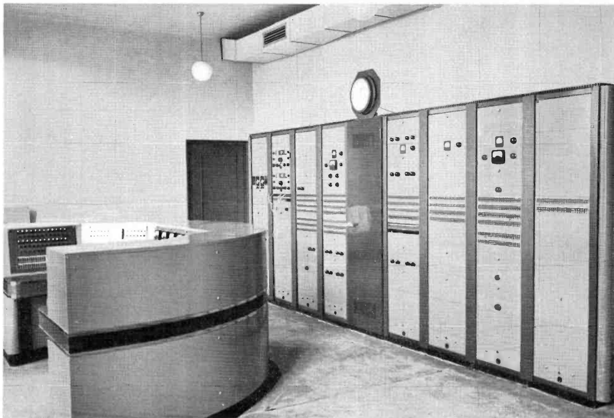
FIG. 11. Another view of the equipment racks and control desk in the studio master control room.
