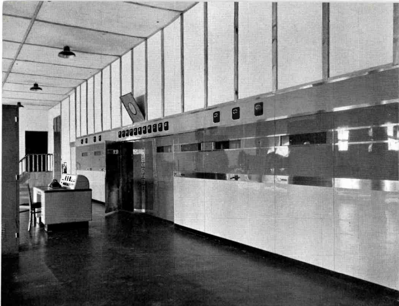
FIG. 1. Front panel of the "Voice of America" transmitter as seen from right side of room.
