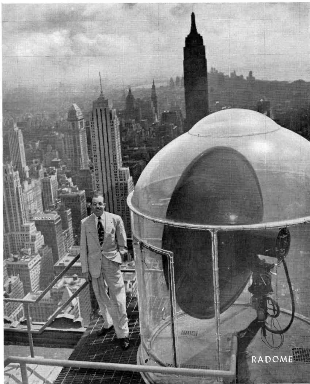
FIG. 2 Special plastic housing, known as a "Radome," protects NBC's microwave relay equipment from high velocity winds and adverse weather conditions often encountered atop the skyscraper RCA building in Radio City. Shown in the picture is O. B. Hanson, NBC Vice-President and Chief Engineer.
