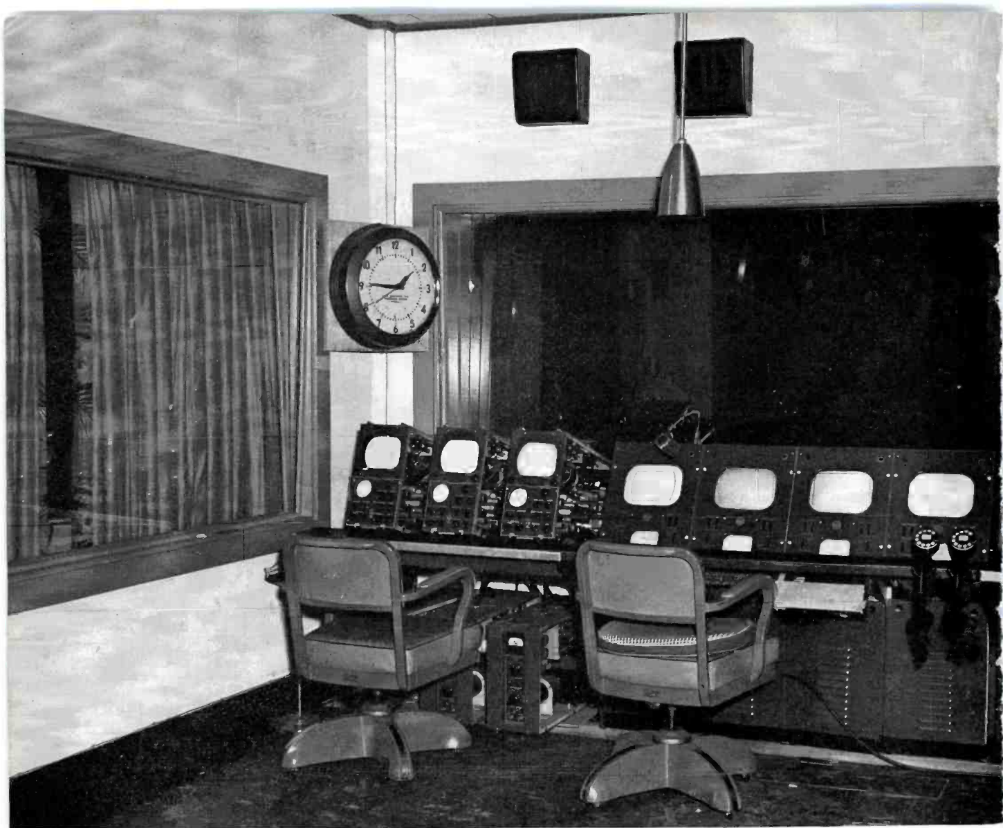
FIG. 7. One side of the studio control room contains (at left) three camera controls for the three field-type cameras used in the studio. Other equipment visible, left to right, includes line monitor and TS-10A Camera Switching System, preview monitor, and two film camera controls. Audio console and equipment racks are not shown. Side window joins clients' viewing room.
