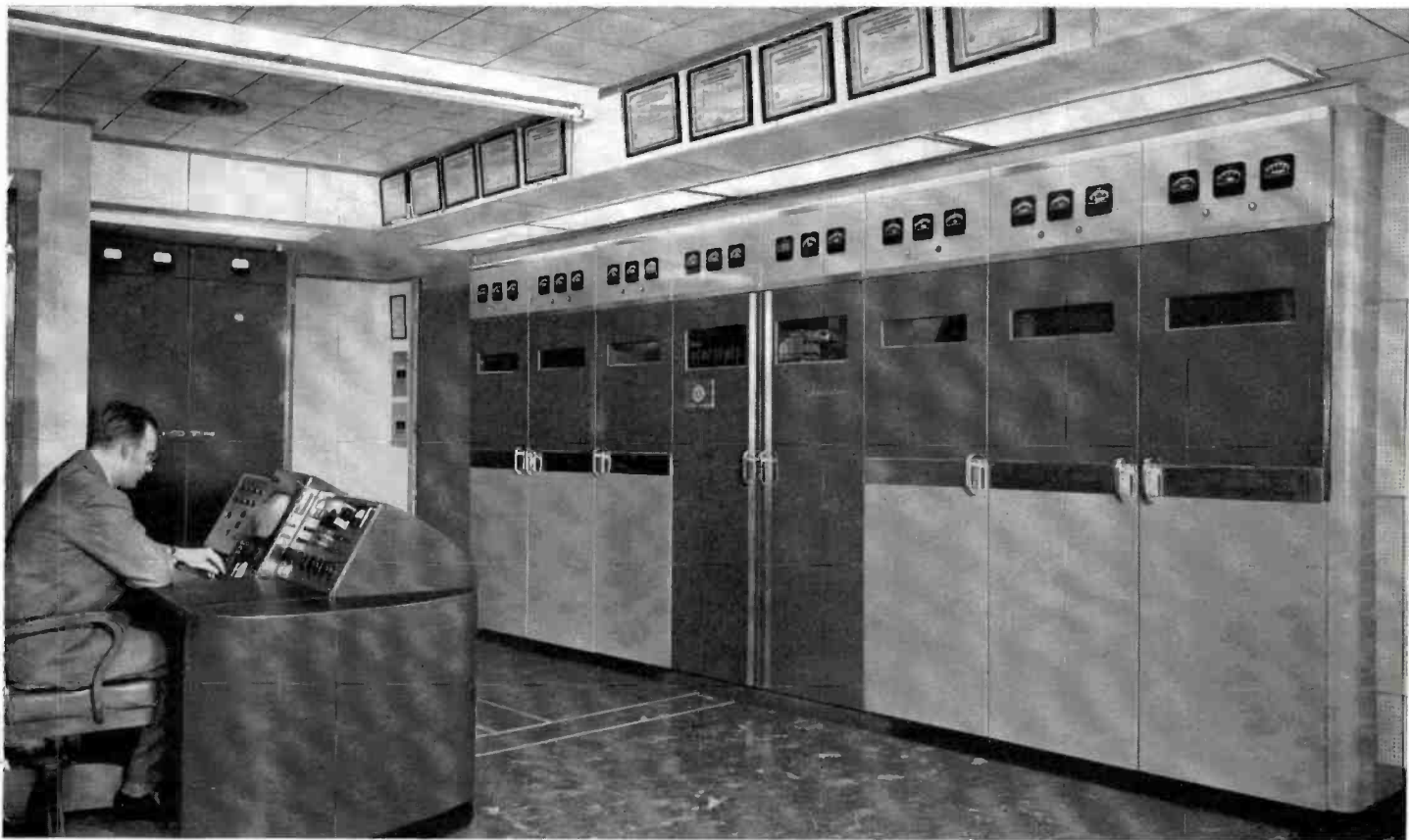
FIG. 3. Mr. Frank Vials, transmitter engineer of WAAM, seated at the console of the RCA TT-5A Television Transmitter. WAAM operates on Channel 13 with an effective 26.1 kw visual power and 13.8 kw aural power. The antenna is a six-section Super Turnstile.
