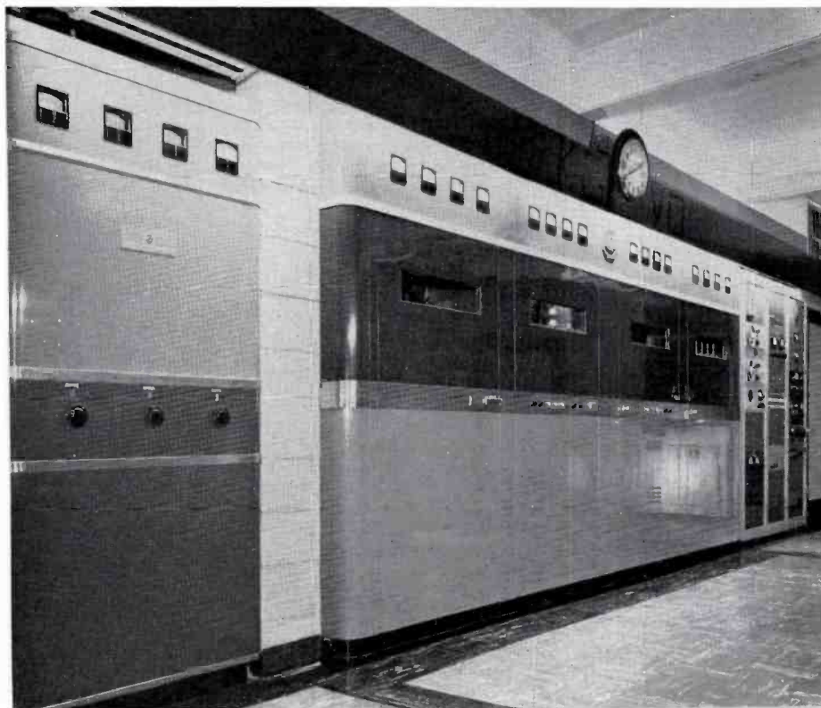
FIG. 2 (below). In this view are shown the complete transmitting equipments; from left, the RCA custom phasing cabinet, the BTA-5F transmitter, and the audio and monitoring racks.
