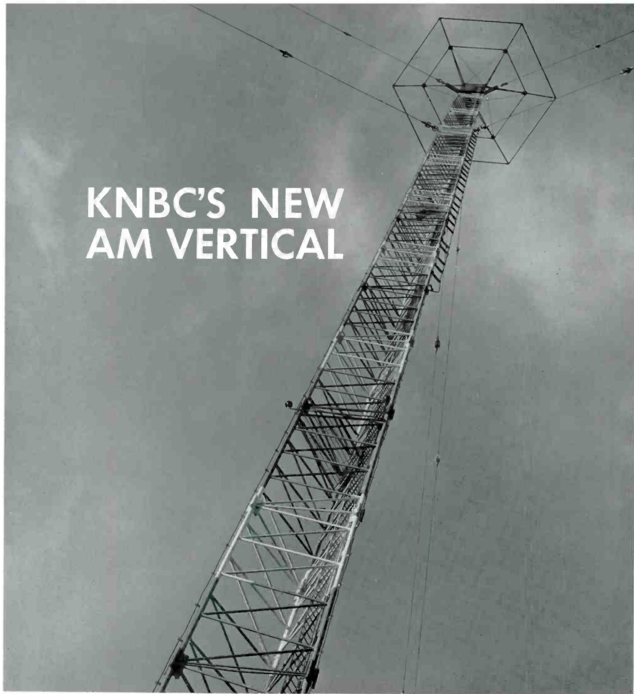
FIG. 1. Dramatic close-up view of the new vertical "articulated joint" AM radiator installed at Belmont. Distance between the upper and lower guy wires is 150 feet. The "articulated" joint is just a few feet above the point of attachment of the lower guy wires.
