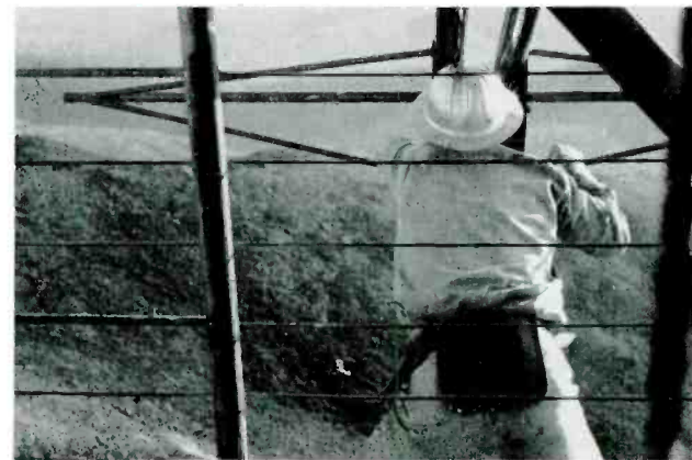
FIG. 13(A). All electrical connections to the antenna were made by erectors under the chief engineer's supervision.
