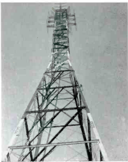
FIG. 3. The KRON-TV Ideco tower and TF-DA three-section antenna which will later be made directional by moving back screens to front side. Note gradual curve of transmission line which follows ladder girls inside tower to eliminate special angle and reduce discontinuity of line.
