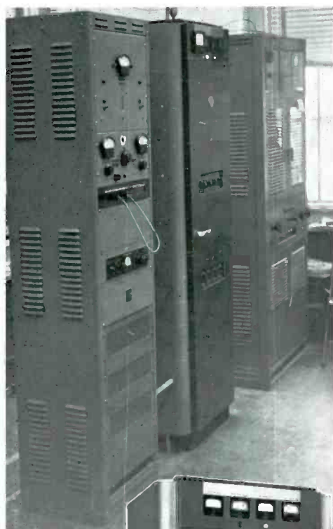
FIG. 1. View of WNAG's transmitter room.
