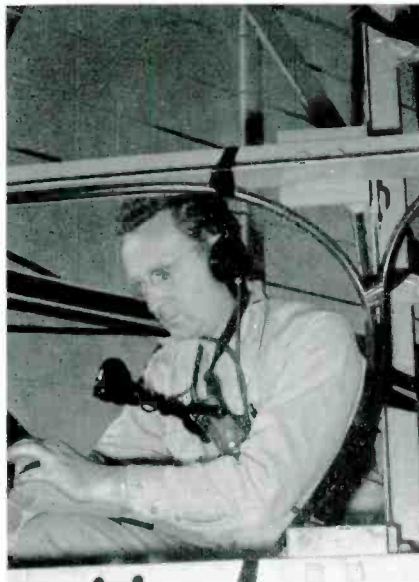
FIG. 11. All work was personally supervised by R. A. Isberg, Chief Engineer of KRON-TV, shown here checking junction box at the center of the antenna. The feed lines were taped to the supporting structures with Scotch electrical tape and then painted with red Glyptal. Aereosal clamps were used to secure the cable to the structure.
