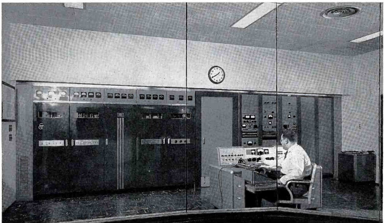
FIG. 17. Front view of the KNBC-FM transmitter and FM monitoring and test equipment at right. All equipment is installed "in-line." Sam Melnicoe is the engineer on duty.
