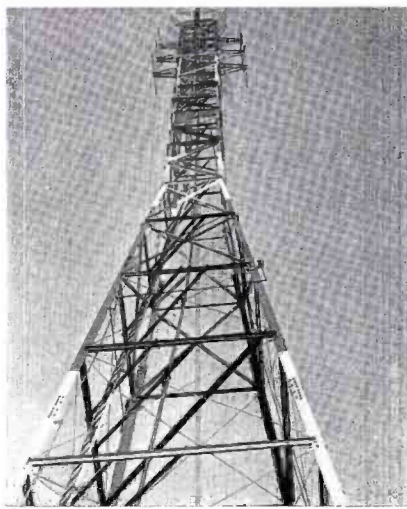
FIG. 3. The KRON-TV Ideco tower and TF-DA three-section antenna which will later be made directional by moving back screens to front side. Note gradual curve of transmission line which follows ladder girls inside tower to eliminate special angle and reduce discontinuity of line.
