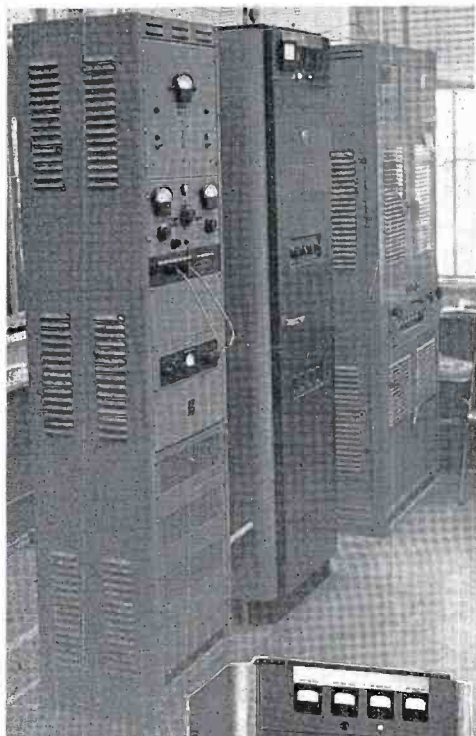
FIG. 1. View of WNAG's transmitter room.
