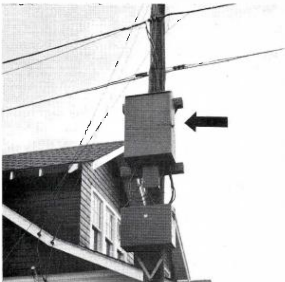
In addition to the main amplifier, line amplifiers like those below are inserted wherever needed to maintain a definite value of signal strength.
