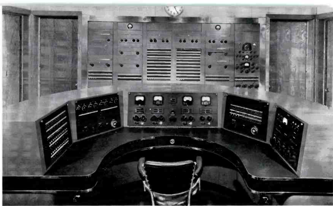
1940 Master Control Console installed at Radio Station WLS. In this arrangement controls, meters and switches are convenient to operator by a "U" type turret arrangement. Audio racks are installed nearby at the rear of console.
