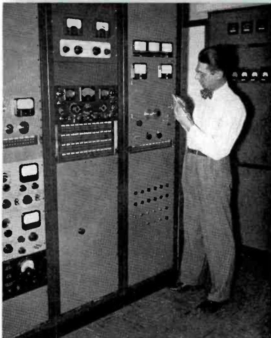
FIG. 5. Mark Boese, KSOO engineer, checks current ratios and phases at Phase Monitor. Push button controls for remotely controlled tuning motors and supervisory lights for the pattern change relays are shown.
