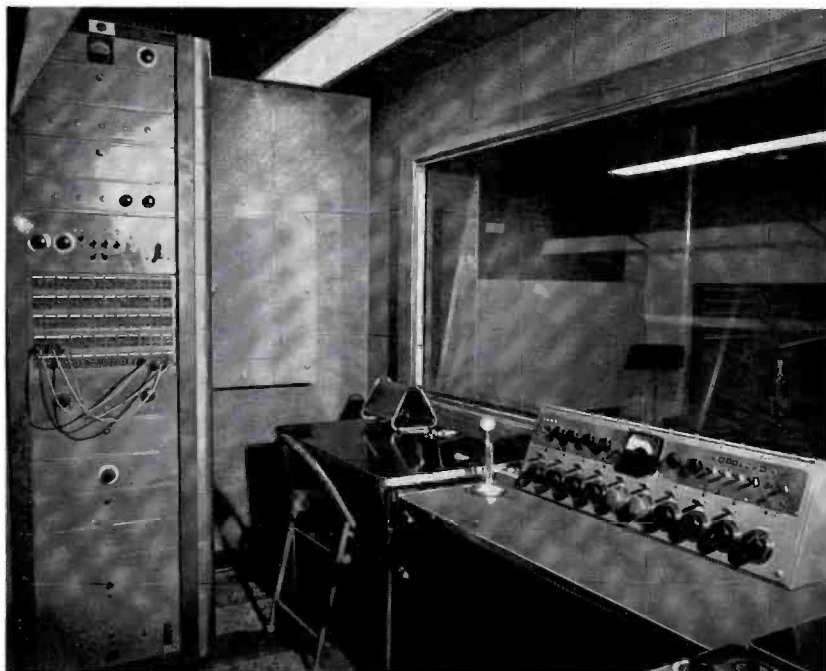
FIG. 7. Studio C's Console has many desirable features for a functional program studio. This RCA Custom-Built Console is equipped to handle four microphone inputs, two turntables, and facilities for remotes 1-2, 3-4, and a network control. A special feature is the Echo Effects circuit built into the console, highly desirable for dramatic programs.
