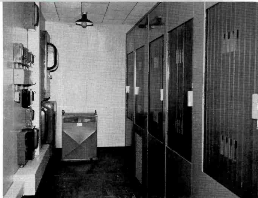
FIG. 6. Rear view of RCA BTA-10G Transmitter installed at KSOO. Power distribution panel may be seen at left. Power transformer for transmitter is shown at the rear center.
