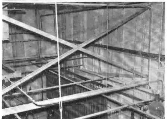
FIG. 49. One system of Cope duct runs around the top of each studio in the Tele-Truss area (middle of the picture at right). Short runs from this duct to fixtures are made with standard conduit. Open top of the duct allows cables to be changed or added very easily.
