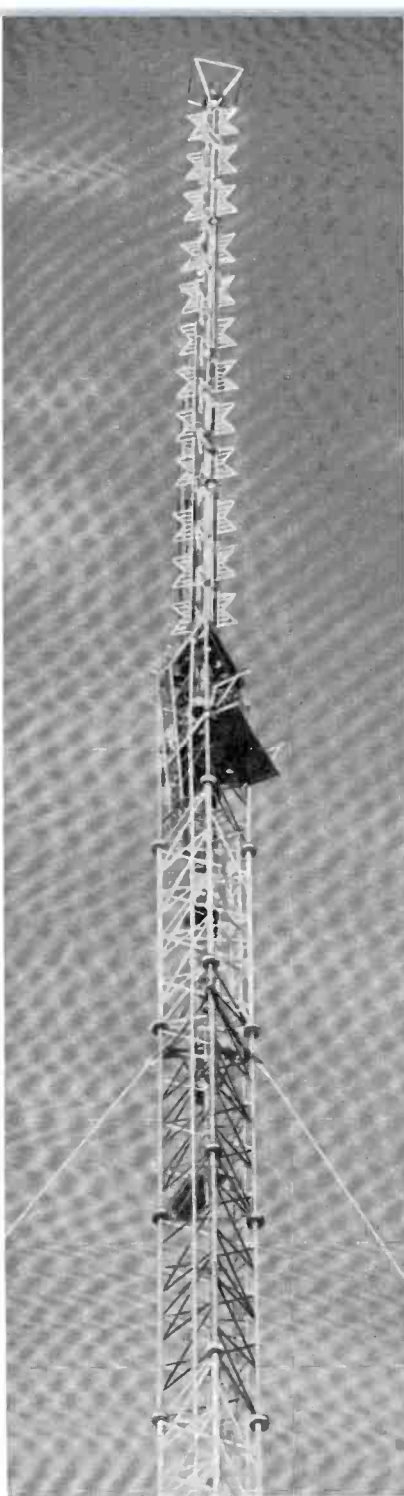
FIG. 5. The completed antenna installation is shown here on its triangular, 500-foot guyed tower. It was erected through the combined efforts of the KTBC engineering staff, RCA engineering, Ideco and the Seago Construction Co., erectors.
