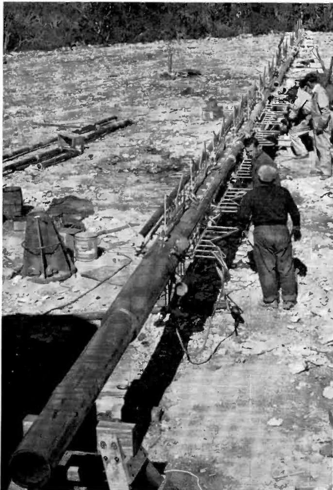
FIG. 1. Ground view of the RCA 12-section Superturnstile high-power, high-gain antenna—Type TF-12AH. Feed lines and transmission line are receiving final check before hoisting.
