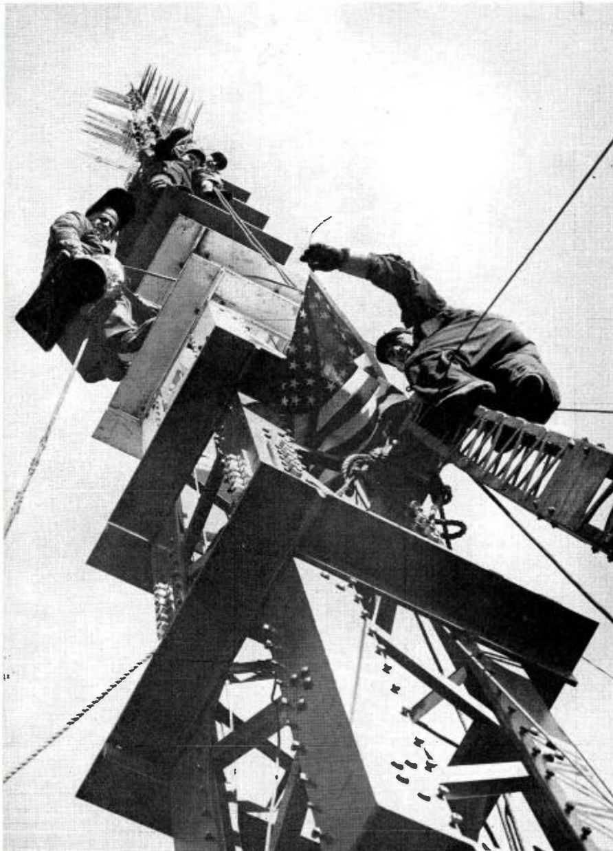
FIG. 4. Photo showing a closeup of the "multiple-use" TV antenna supporting tower located atop the Foshay Building. The seven diaphragms on lower portion are for strengthening and permit supergain elements to be mounted in between them.
