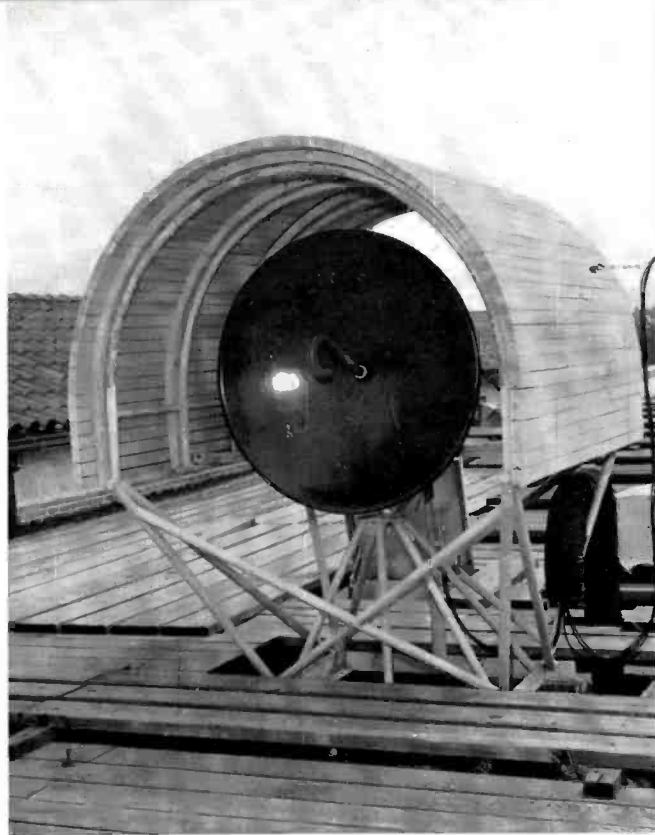
FIG. 24. WBAP has two microwave relay pickup points: one is this parabola on the roof of the studio building, another is on the Medical Arts Building in downtown Ft. Worth.
