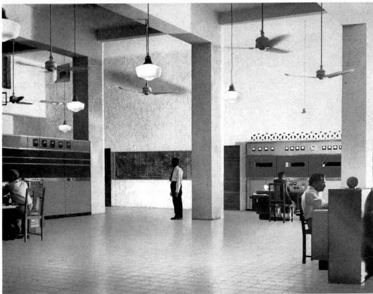
The spacious Transmitter Hall is equipped with two RCA 50 kilowatt, dual-channel, high frequency broadcast transmitters and one RCA 10 kilowatt medium frequency broadcast transmitter. The building has been designed so that additional equipment may be installed and additional construction carried out for future expansion.
