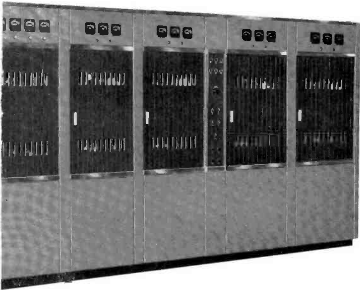
RCA's newest high-power television transmitter (Type TT-25A) which will be installed in WBAP-TV's new transmitter building in the near future.
