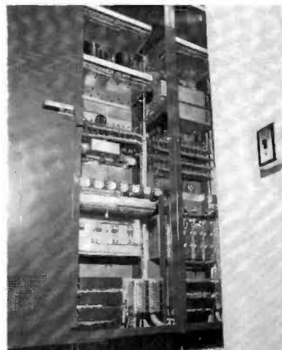
FIG. 10. This rear view of speech input equipment demonstrates the adequacy of jacks which increase flexibility of operation. The neatness of wiring also is apparent.
