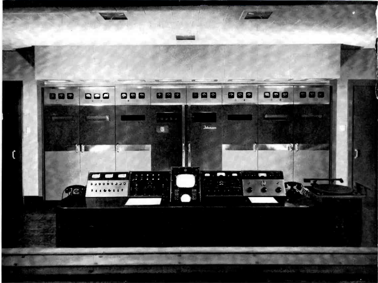
FIG. 17. WBAP's RCA TT-5A Television Transmitter as seen through the window from the corridor which runs the length of the TV area of the building. The control console contains the operating controls for both the TV and the FM transmitters.
