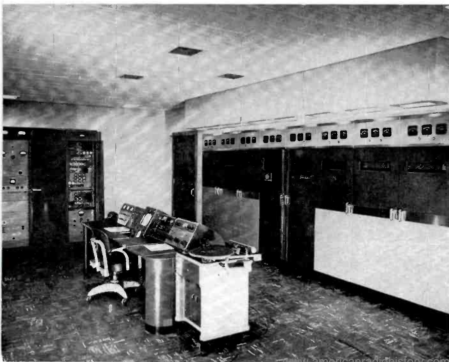
FIG. 18 (below). View looking toward the TV end of the transmitter room. The three cabinet racks at the far end house the television amplifiers, monitors and the auxiliary equipment.
