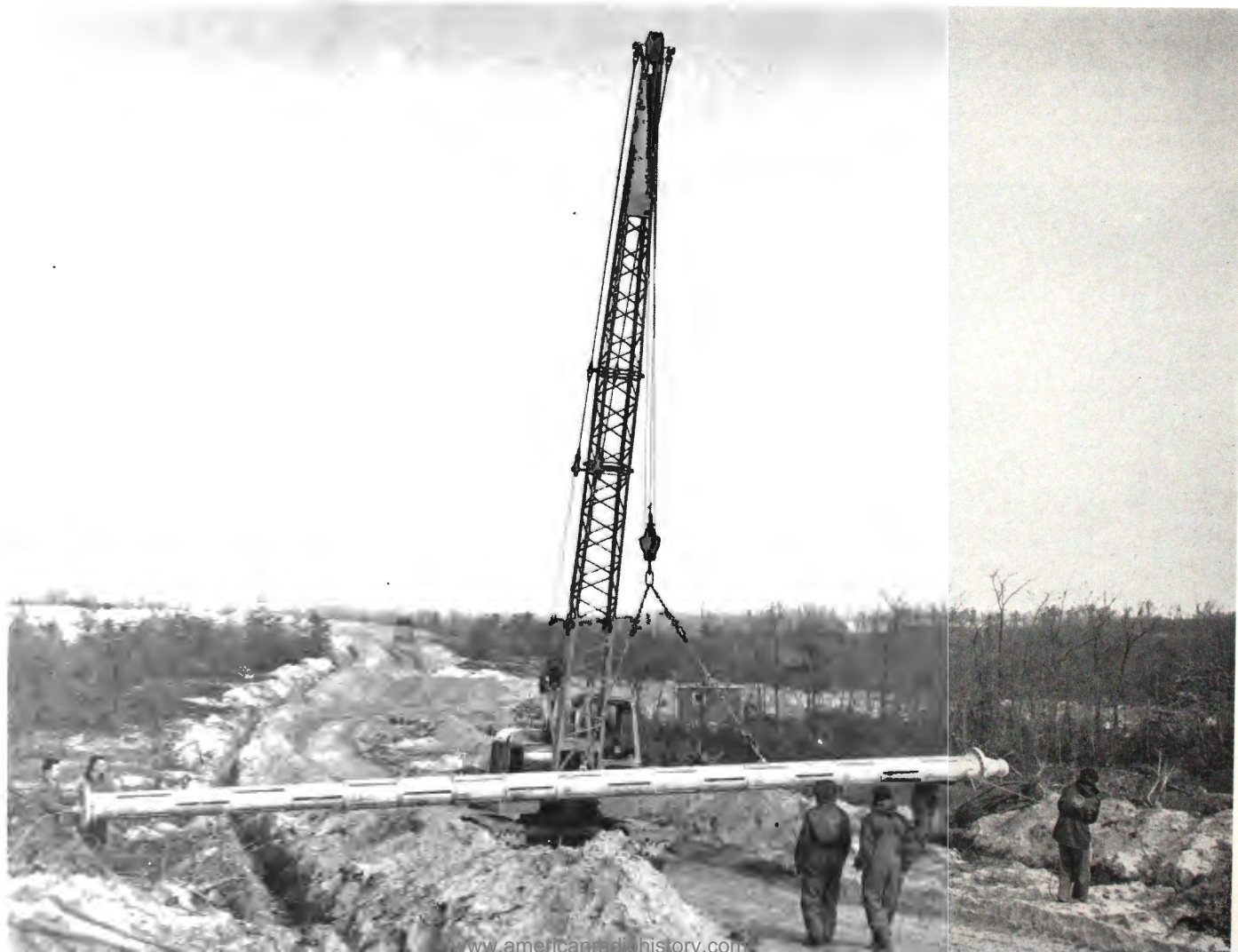
One section of the fabricated antenna is moved up a newly bulldozed road to the Gibbsboro site.
