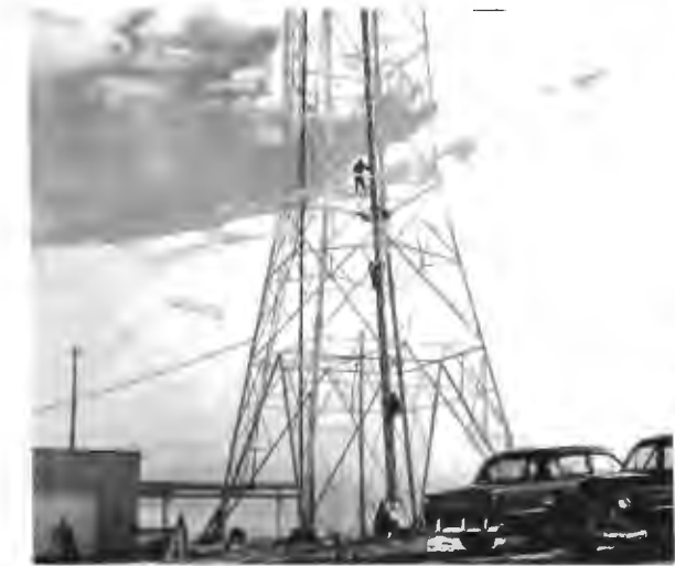
Completely assembled ultragrain Pylon is suspended in the center of the TV tower.
