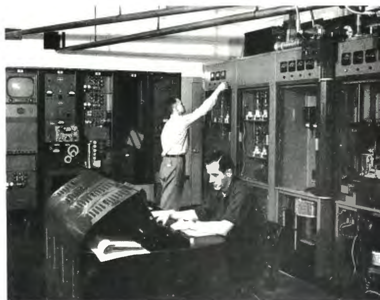
View of the WBRE-TV transmitter room. Four of the TTU-25A Amplifier cubicles are shown at the right. The station's original TTU-12A transmitter (not shown) is placed parallel to these cubicles about six feet to the front of the supervisory console. Transmitter equipment cabinet racks are pictured at the far end of the transmitter room.
