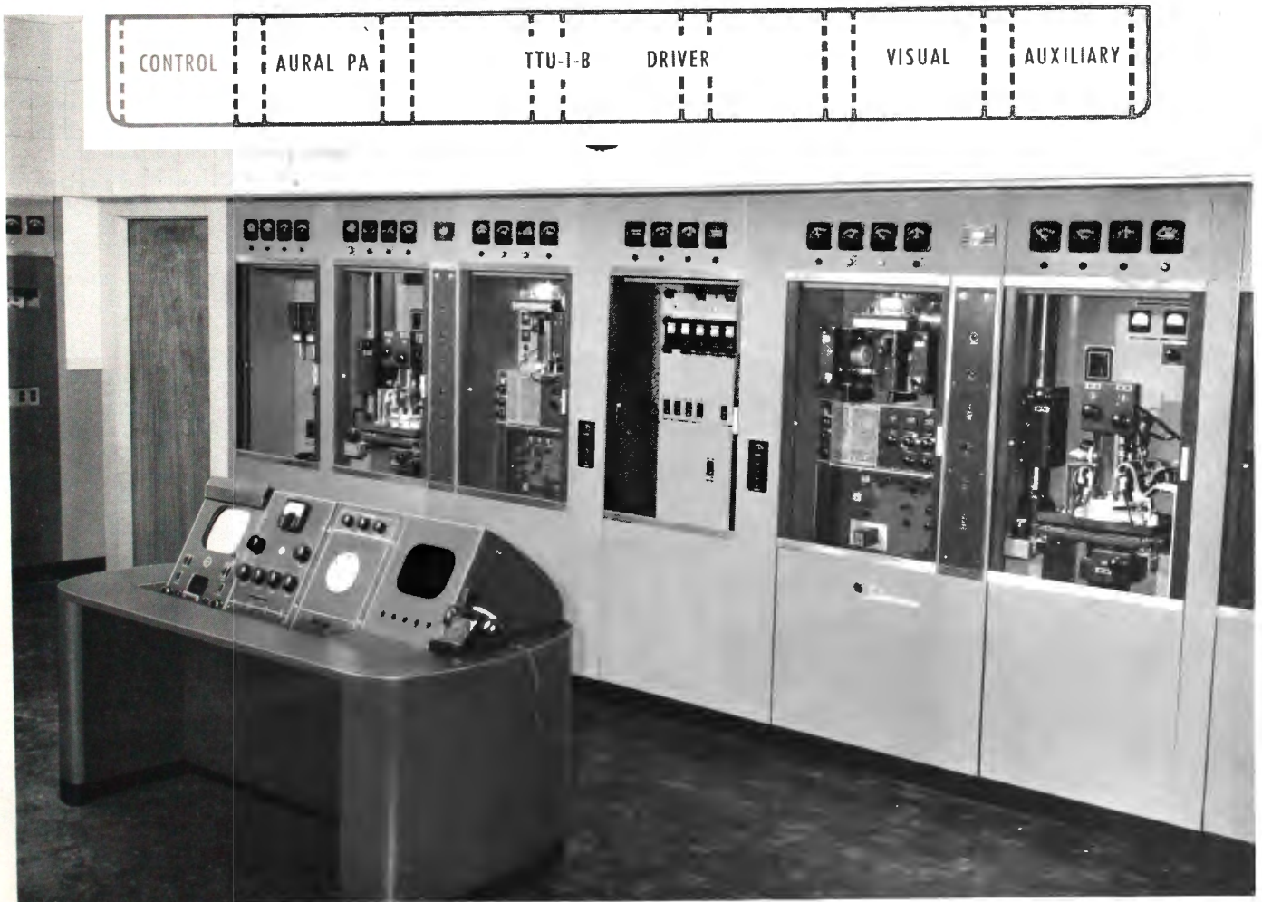
WBRE-TV's original TTU-12A Transmitter. The unit required slight modification in the aural P.A. so that this cabinet now provides the peak aural signal required for 25 kw operation. This transmitter serves as the driver chain for the amplifier pictured on the left hand page. Note that the TTU-1B is still an integral part of the new equipment.
