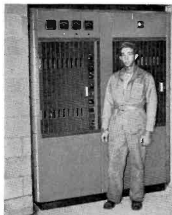
FIG. 6. Shown in front of the BTA-1M and the phasing cabinet, is Tom McFerrin, chief engineer of WCBI, who supervised the complete installation of the new kilowatt plant. The two cabinets will be framed with moulding around the edge of the opening to form a perfect installation from standpoint of convenience and appearance.
