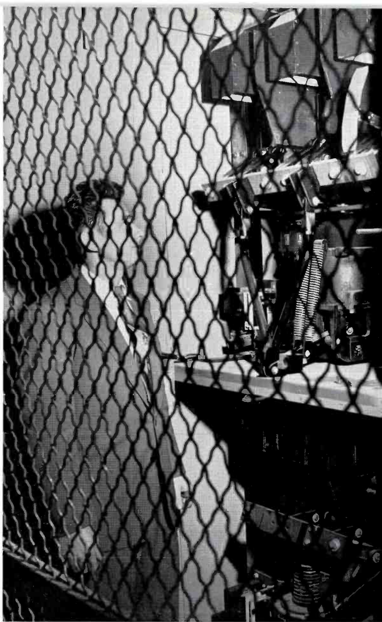
FIG. 8. Jay Cleaves, Building Chief Engineer, shows 3000 amp. and 2000 amp. main electrical breakers with fronts removed.
