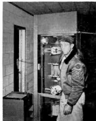
FIG. 7. Tom McFerrin, chief engineer for WCBI and The Mid-South Network, inspects the phasing gear before sliding phasing cabinet into position beside the BTA-1M 1 kilowatt transmitter at the WCBI transmitter.
