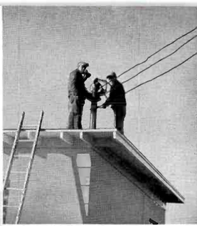
FIG. 1 (left). Power crews connect power to the WCBI transmitter building preparatory to installation of the "all RCA" installation of radio and TV for WCBI. The new site is four miles northeast of center of Columbus, on Highway 12.
