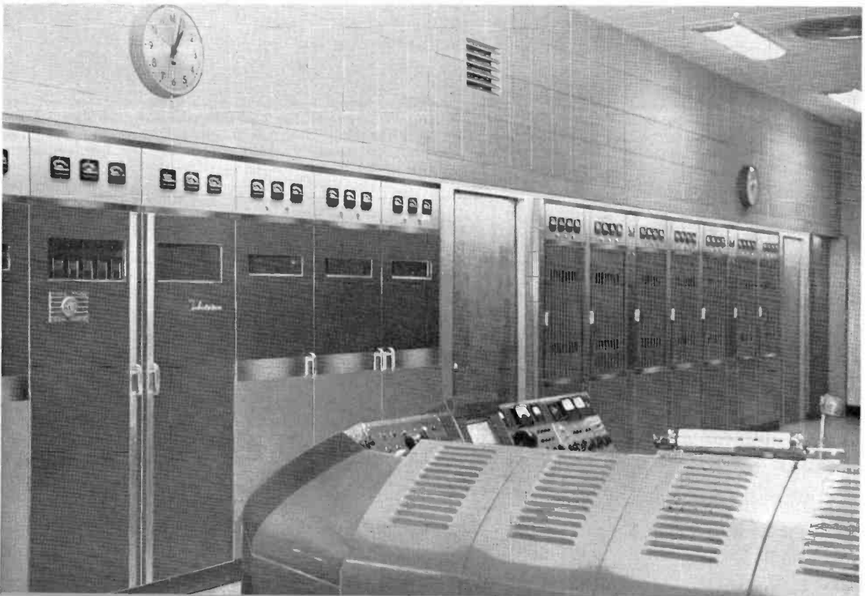
FIG. 29. TT-5A standby transmitter on the left and high power TT-50AH on the right are both monitored by one control console. TV master control extends to the lower right.
