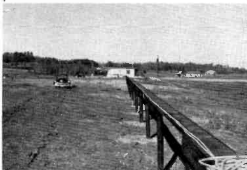
FIG. 8. Creosote-treated raceway from the WCBI transmitter house to tower #3 shown in this view carries the transmission line, power cable, supervisory wires, sampling lines and communication wires between the towers and the transmitter house.
