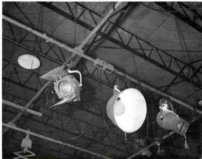
FIG. 17. Part of light grid in studio to show unique conduit construction that supports lights and also carries wiring.
