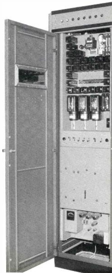
FIG. 6. Control unit is shown with door open. Auxiliary switches are located on the panel in the center. Above this panel are all the overload relays as well as the auxiliary relays associated with the overload recycling circuit.
