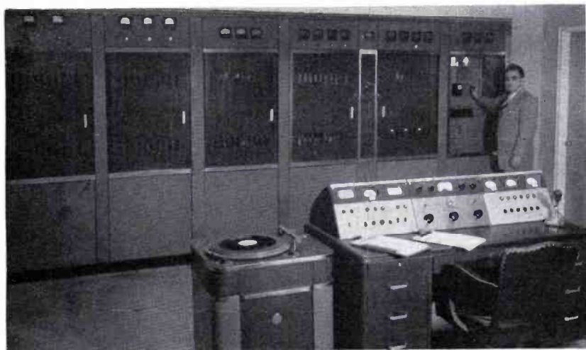
FIG. 5. View of BTA-5H AM transmitter and console. Two cabinets at left are phasing equipment. Right-hand console turret contains control for switching each of the three AM transmission lines to a spare line. Engineer in picture is B. J. Weimer, Transmitter Supervisor.
