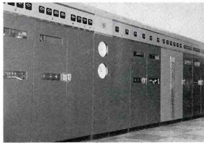
FIG. 11. At transmitter center in Germany nine broadcast transmitters are used. Shown here is part of two RCA 50-kw transmitters used in this area.
