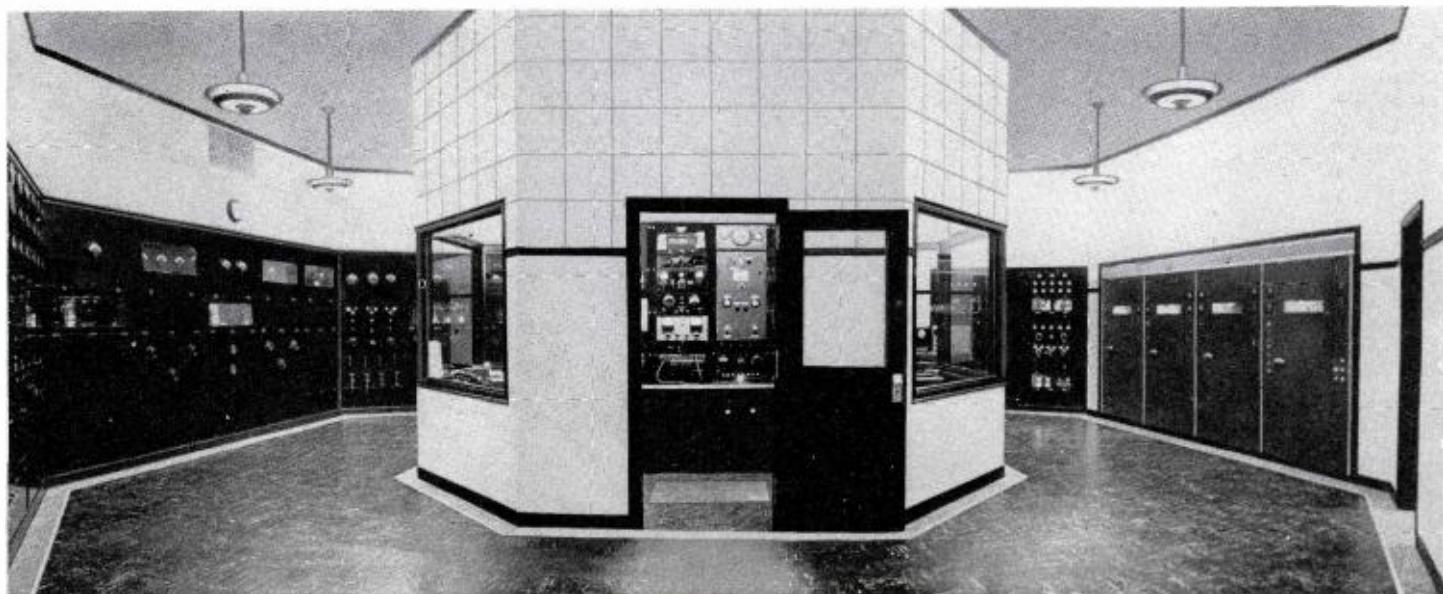
FIG. 1. Interior of transmitter building at KSTP looking toward the rear of the octagonally shaped room. At the far right, the four cubicles of the BTA-50G 50 KW AM Transmitter can be seen. Just to the left of the BTA-50G is a composite 1-kw stand-by transmitter housed in two cabinets. The control room at the center of the main transmitter room contains the transmitter test and measuring equipment as well as facilities for programming of records and station breaks. At the left of the control room, a portion of the old composite 50-kw AM transmitter can be seen. This composite 50-kw unit takes up approximately one-half of the wall space of the transmitter room. In contrast to this, the new BTA-50G occupies less than 15 feet of wall space—an area formerly occupied by a 10-kw FM transmitter.
