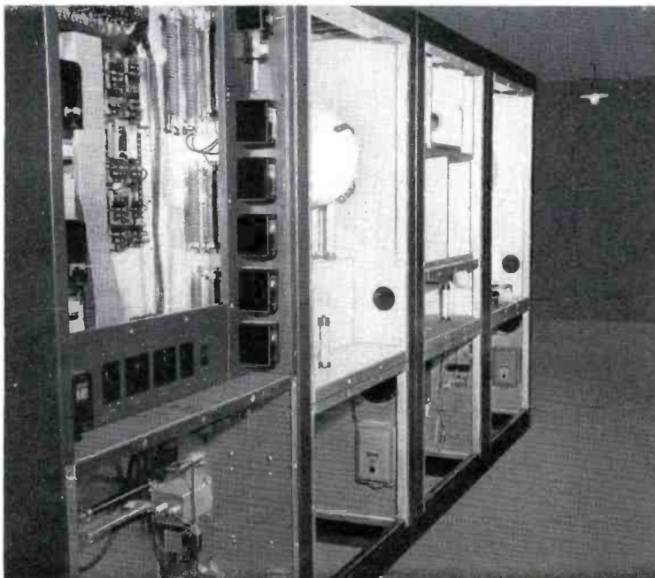
FIG. 4. Rear view of BTA-50G shows transmitter during installation. Bottom sections of frame are removable to allow heavy components such as the filter reactor, blowers and low voltage plate transformers to be moved into place.
