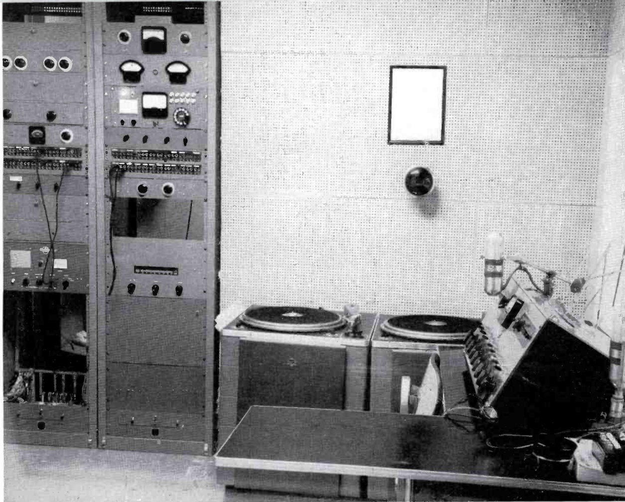
FIG. 3. Complete equipment facilities in Control Room A include a BC-2B Console, two BQ-2A Turntables and two equipment racks.
