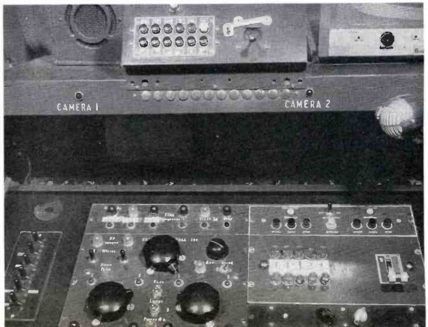
FIG. 15. Closeup of WISH-TV subcontrol console showing Technical Director's position. At top is control panel for video effects equipment. Keys at left for plant intercom. Center panels for remote control of monochrome projector No. 3, slides, and opaques. Right hand panels from top to bottom: projector controls for color projectors, TS-5 switcher, and switching panel (black and white knobs) for connecting video into effects equipment.
