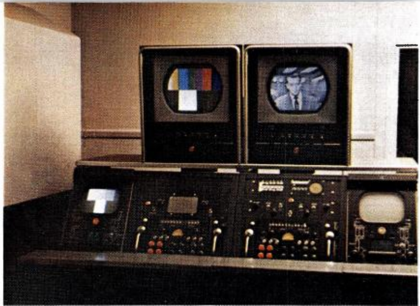
FIG. 36. TK-41 color camera control room console consisting of monitors and control equipment for two live color cameras. This room also contains an equipment rack housing the two colorplexers associated with the cameras. Windows opening out into Studio B at the right.
