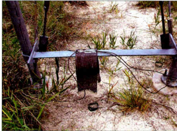
This ground strap, on the last Ice Bridge before the building, should be cut.
