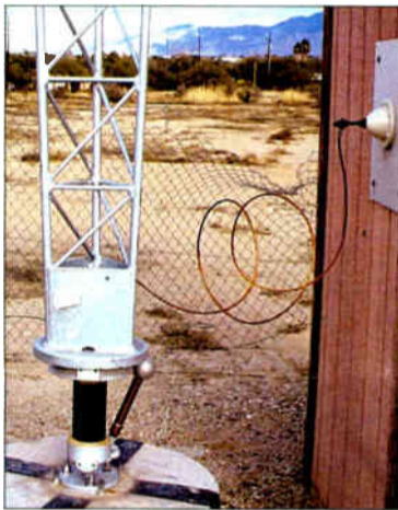
Coiling conductors provides an inductive path against strikes.
