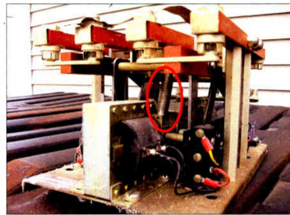
The Cardwell contactors would fail when this part broke apart.
