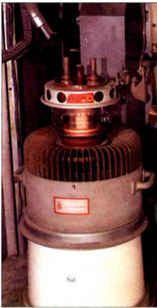
One of the 5671 PA tubes in its socket.
