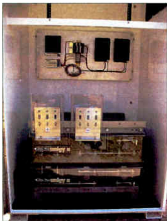
The 12 VDC, 1470 amp-hour modular AGM battery iPowerPV batteries and pre-assembled solar electronics. The 19" rack for customer equipment is located at the top of the enclosure.
