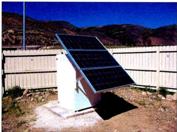
Solar modules after installation on a three-module iPowerPV.
