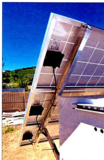
Wiring the solar PV modules after they are mounted on integrated aluminum rack assembly.
