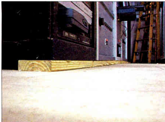
Wooden blocks insulate the equipment from the circulating currents.
