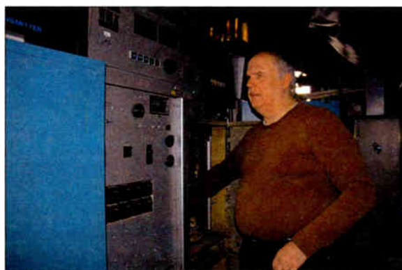
Stachowiak checks out the PA cavity in WBLK’s RCA FM auxiliary transmitter.
