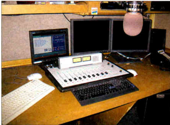
KMYK's on-air studio with the new Arrakis ARC-10.
