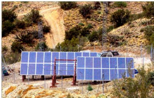
The Solar Panel Array in the Rough Terrain
