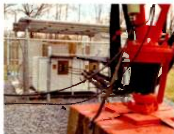
AM Cellular Colocation
