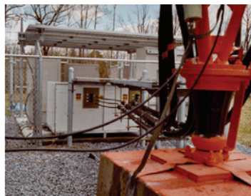
AM Cellular Colocation
