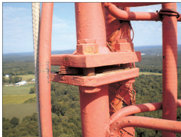
Flange with Only Two Bolts and Shims
