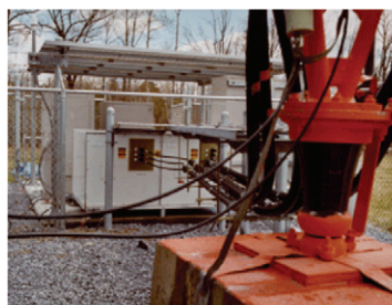
AM Cellular Colocation
