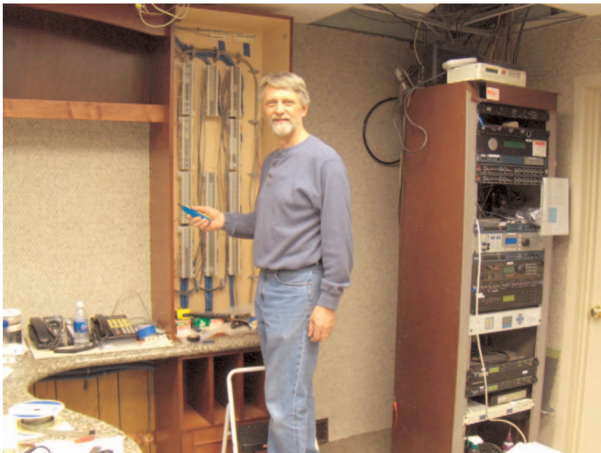
Scott's Wire Closet
