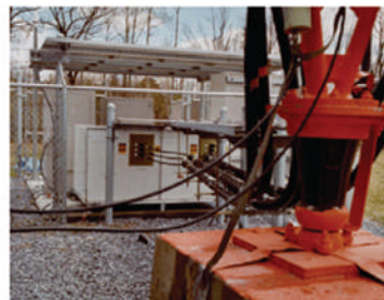
AM Cellular Colocation
