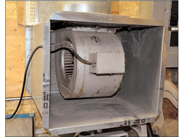
Scott's home brewed intake blower.
