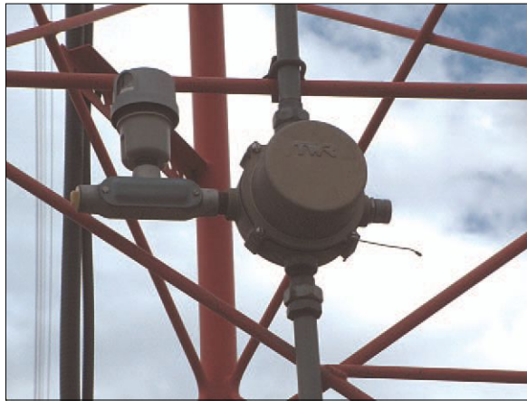
Junction Box and Photo Eye. (Photo 1)
