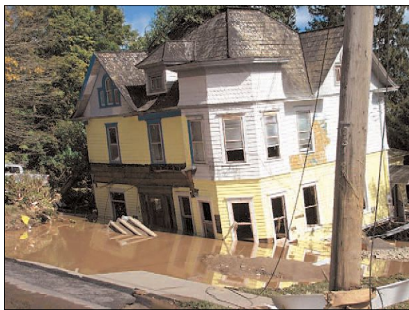
A house knocked off its foundation in Prattsville, NY.
