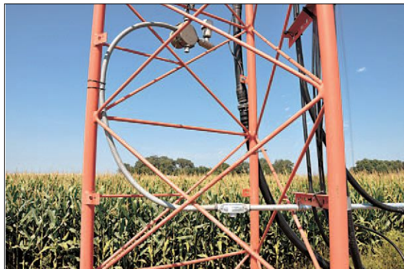
The finished project with flex conduit, and the drain hole facing down to allow proper drainage.
