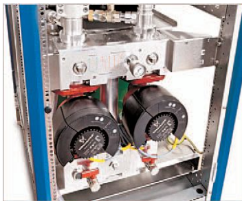
Coolant Pumps in the Rack
