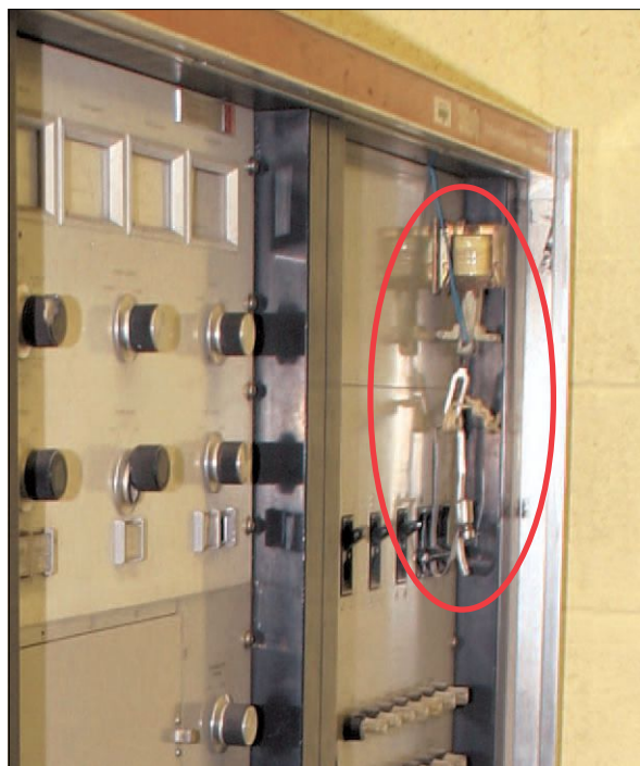
Solenoid to Reset Plate Breaker
