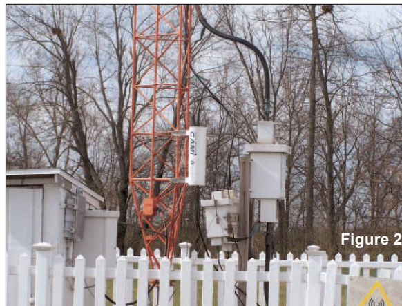
Multiple FM and TV translators in Illinois collocated by an LBA CAMI®500 and two KTL FMC isocouplers.
