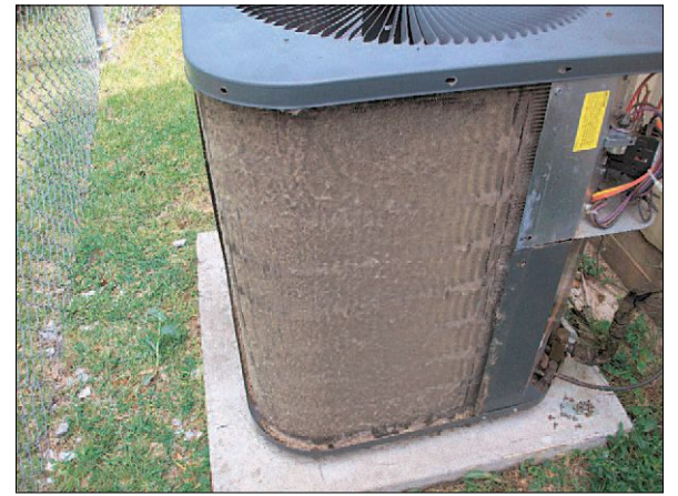
AC Condenser Units Can Become Easily Clogged
