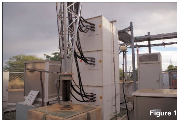
LBA ColoCoil® AM tower collocation in Hawaii, with 12 coaxial cellular antenna feeds.
