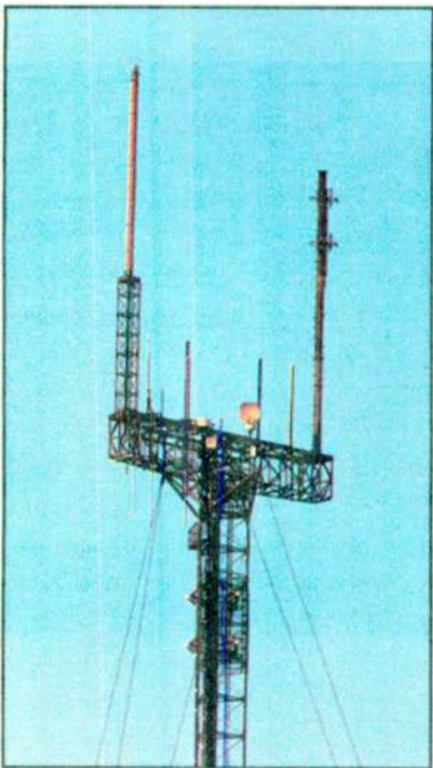
RF chains will be part of the NAB workshops.
