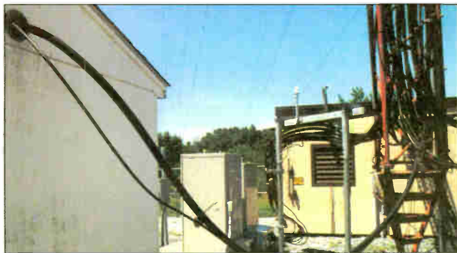
Fig. 2: An ice bridge will also provide cable support
