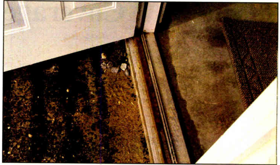
Fig. 3: Inspect transmitter building doors for water damage.
