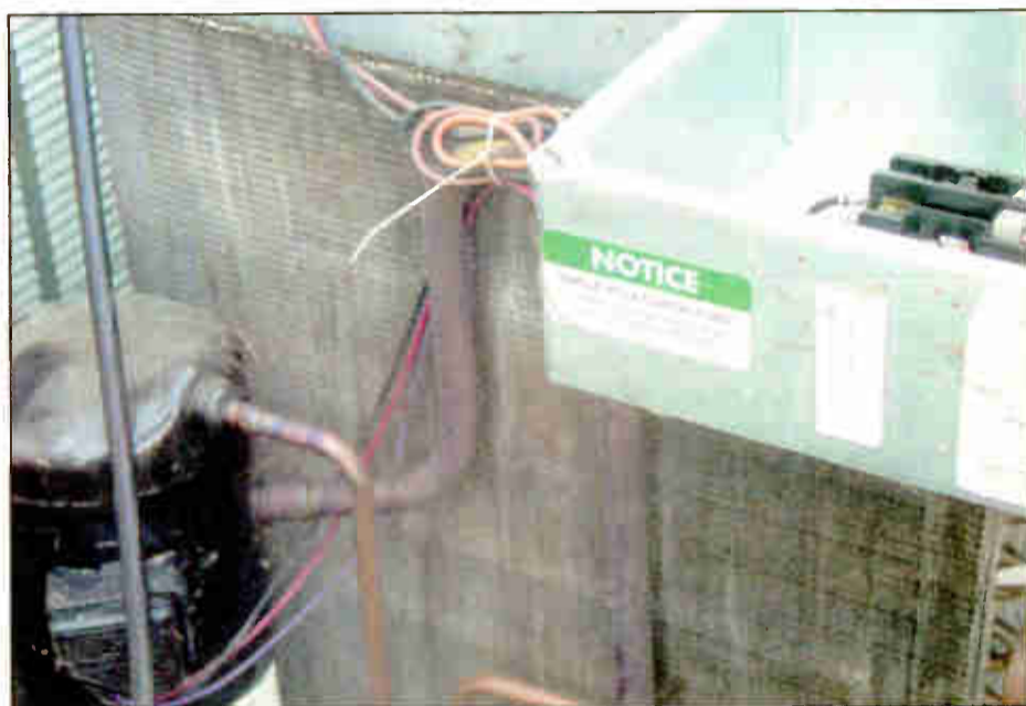
Fig. 2: Dirt inside the heat transfer fins of a compressor/evaporator can impair air-conditioning efficiency.
