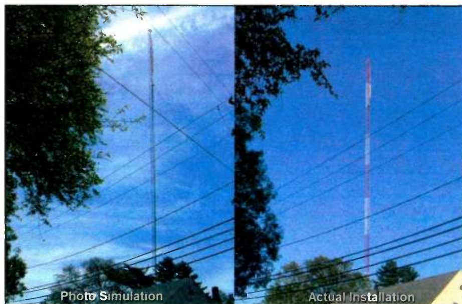
Fig. 1: Image at left shows simulation of proposed antenna before construction as part of exhibit for zoning board. At right, actual tower construction.
