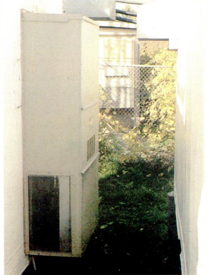
Bard Wall-Mount Air Conditioner Installed on Transmitter Container
