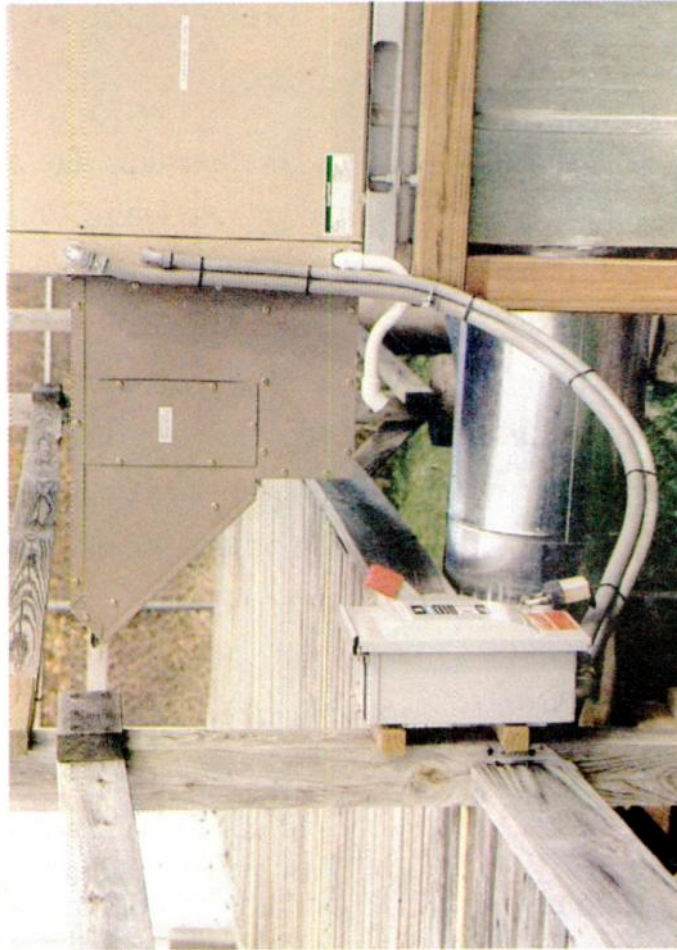
Outdoor Condenser Unit with Electrical Disconnect
