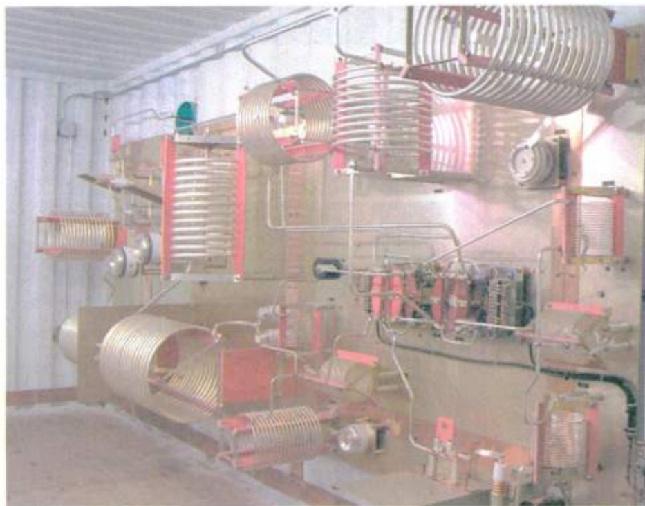
WBIX Phasor at WAMG Five-Tower Array
