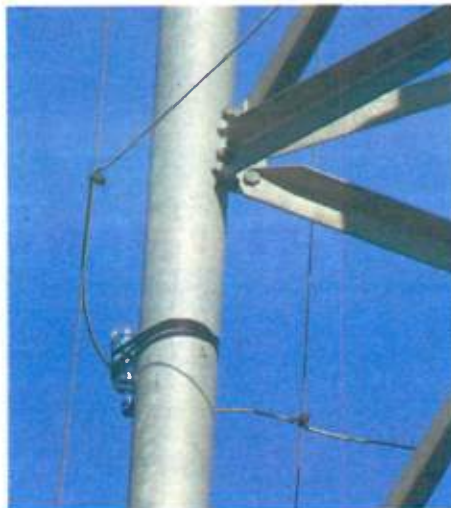
Fig. 4: A plastic bottle prevents arcing until a suitable replacement can be installed.
