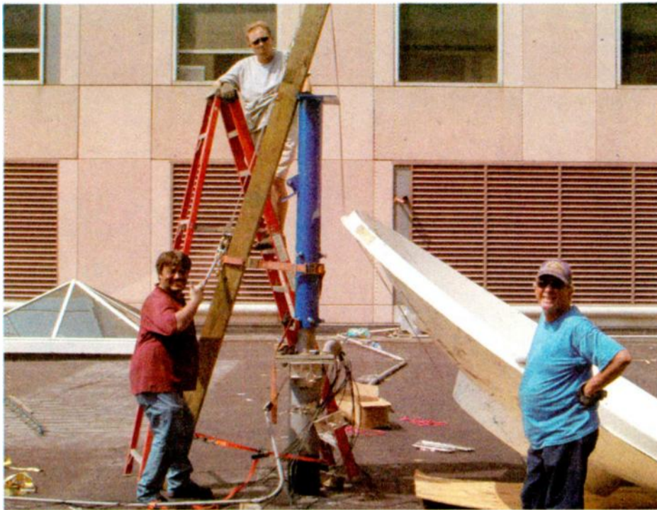
Crew sets 3.8-meter dishes on rebuilt mounts on a rooftop at WWL in New Orleans, in this photo provided by Michael Patton. 'Note the improvised gin-pole used to raised the heavy dish into position,' he wrote. 'All the old dishes and their mounts were destroyed and scattered in the storm; one mount lay on the ground between the building and the sidewalk for almost six months before anyone got around to salvaging it. I would not have wanted to be there when that 400-pound mount went flying.'
