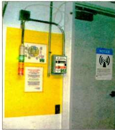
Fig. 10: Alerting light system is installed at each roof access and tower access point at the 4TS facility. The lamp status controlled by the RECON system controls the message that is played by the TowerSwitch enunciator system located adjacent to the alerting light.
