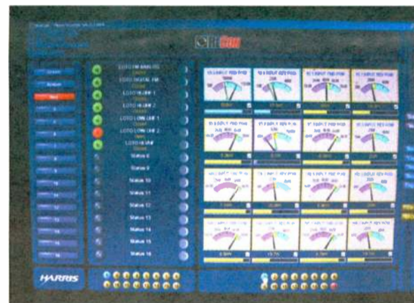
Fig. 9: CRT display of the Harris RECON system used for continuous monitoring of the status of each transmitter at the 4TS facility. Trip points may be set to cause activation of alarms based on transmitter power levels.
