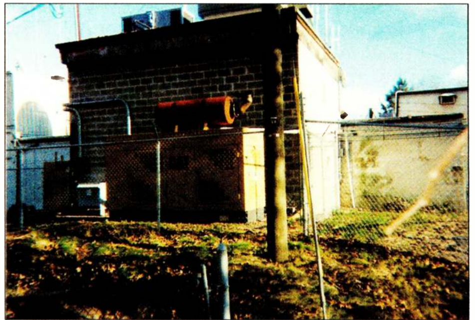
Generator for Backup Power Shown Installed in Outdoor Enclosure
