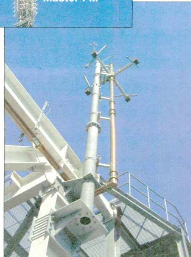
Fig. 3: Close-up photograph of the Lindenblad FM backup antenna at the 4TS facility mounted to the steelwork of the eastern-facing 4TS sign.
