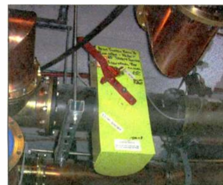
Fig. 12: A manual patch is used to isolate the main combiner feed from either the main or backup antenna. The lock-out/tag-out switch preceding the patch assures that there is no RF energy present, before the patch can be pulled and moved.
