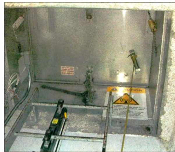
Fig. 8: RF Tower Caution sign installed on tower access hatch.
