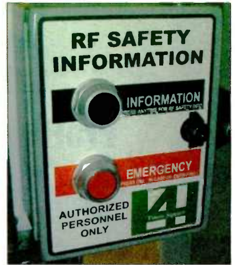
Fig. 11: Close-up photograph of the TowerSwitch RF safety door enunciator unit that is mounted at main roof-access doors, outside on the main roof, and at the hatch and door access points for the antenna tower.
