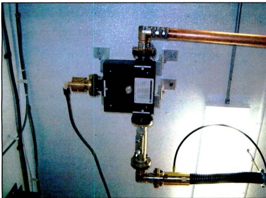
Fig. 8: View of circulator installed on digital transmitter for improved isolation.
