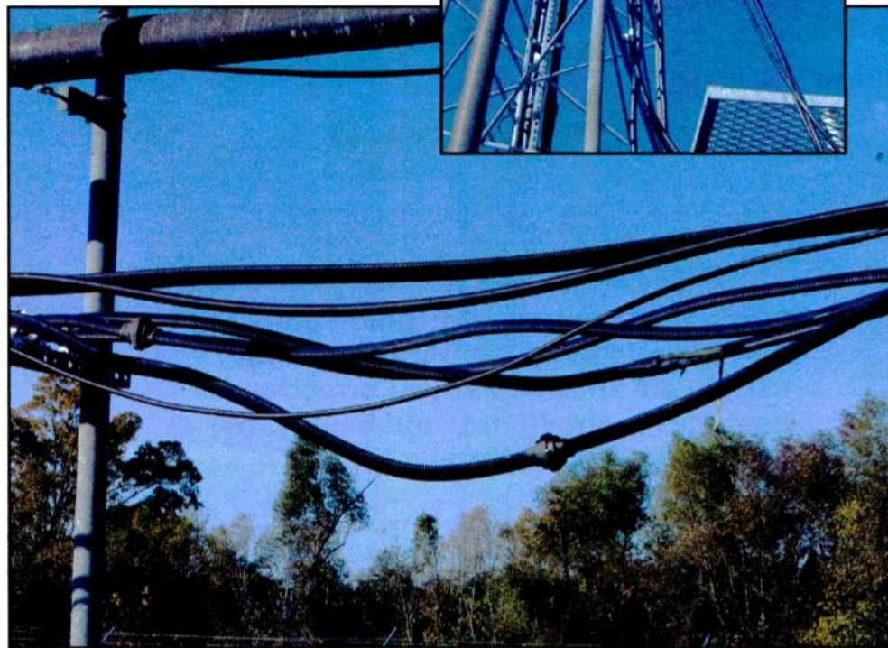
Figs. 7 and 8: Coax cables hanging loosely on the tower need to be fixed. A strong wind can make them act like a whip and bring down the other appurtenances on the tower.
