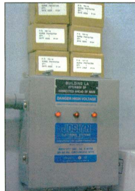
Fig. 4: Be prepared with spare fuses and surge suppressors inside the building.
