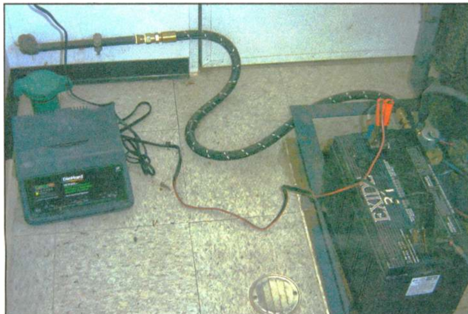
Fig. 1: Batteries and chargers should be checked regularly and should not be lying on the floor.
