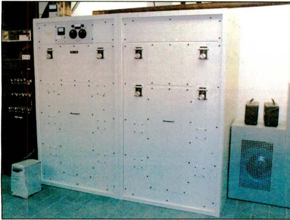
The phasor, where many a night was spent making adjustments.
