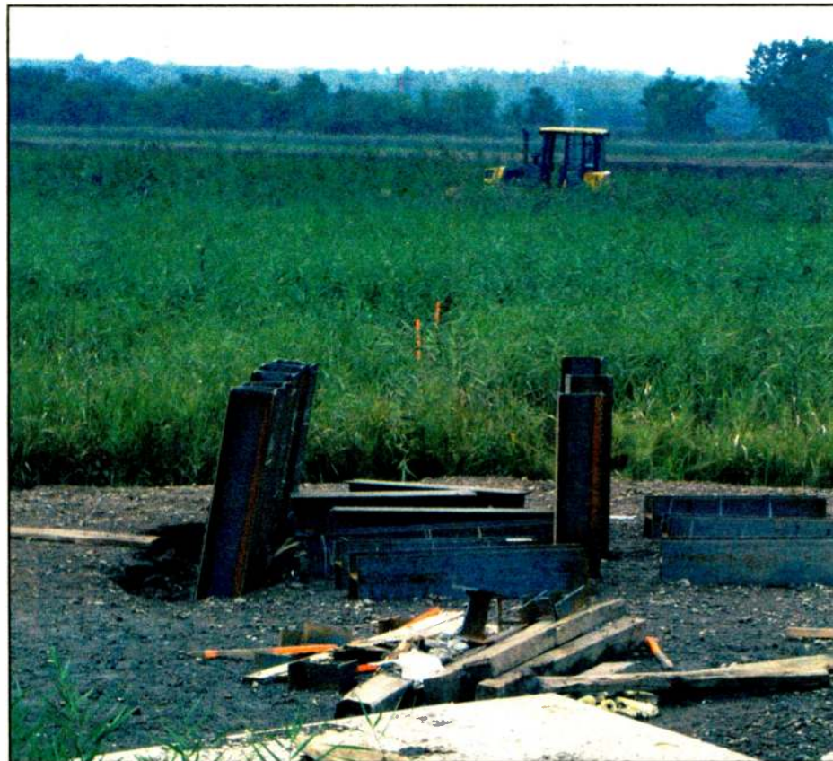
A guy anchor location. Note the angled piles on the left, toward the direction of guy wire pull.
