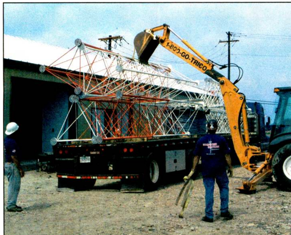
Workers from Northeast Towers remove sections of Tower 2 from the delivery truck.
