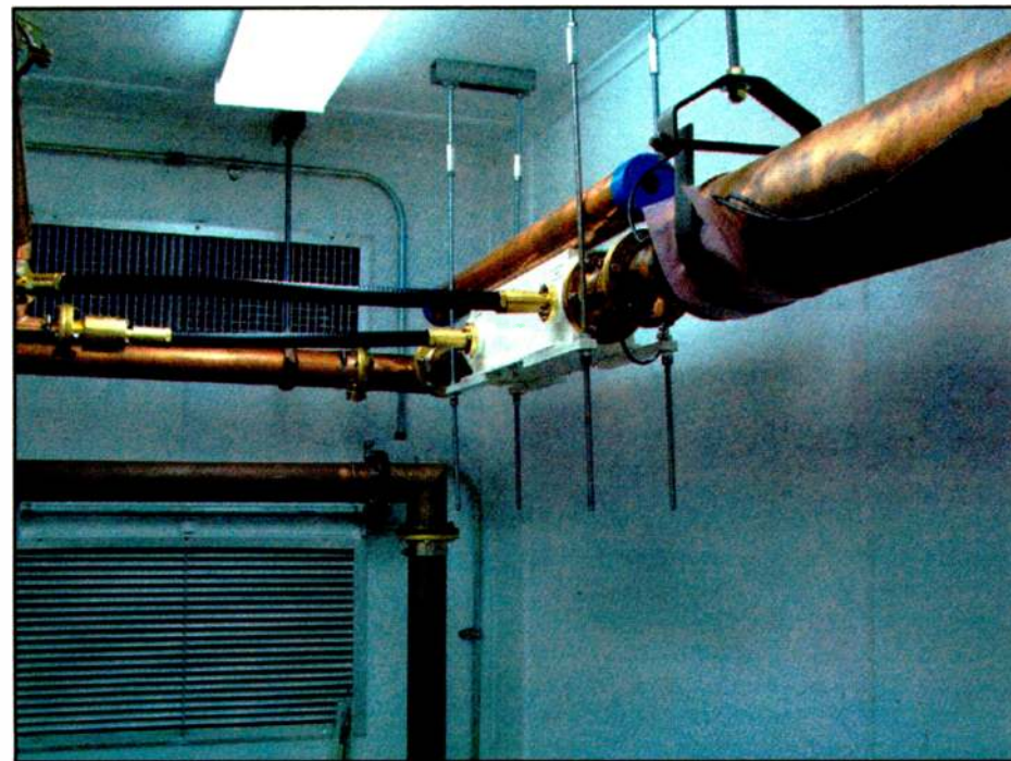
Fig. 1: We found the original 10 dB injector supplied by the transmitter manufacturer to be undersized.
