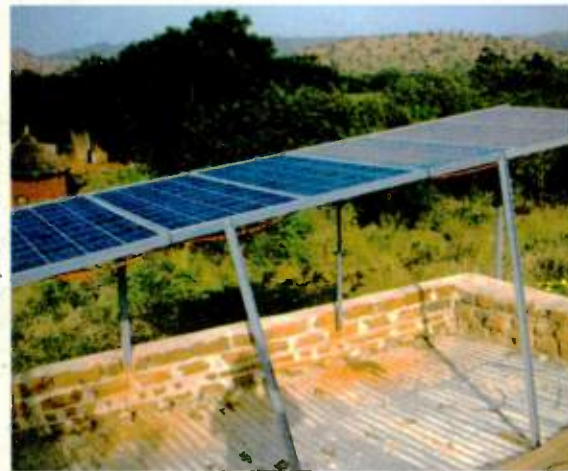
Solar panels help power the station Voice of Community in Kauda.
