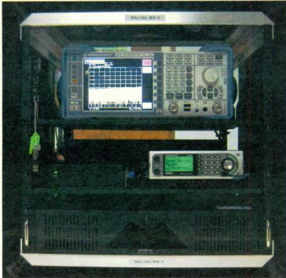
In his presentation, Joe Casey, associate bureau chief of the FCC's Public Safety and Homeland Safety Bureau, discussed the Project Roll Call equipment which includes a Rohde & Schwarz FSL3 spectrum analyzer (top shelf); an ICOM PCR2500 receiver (middle, left), a Uniden 996 scanner (middle, right) and a computer (bottom). The gear is mounted in a shock-protected box.
