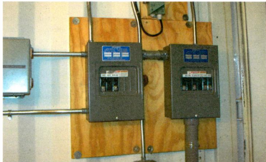
Fig. 2: After replacing the main disconnect fuse, turn on each sub panel breaker one at a time.
