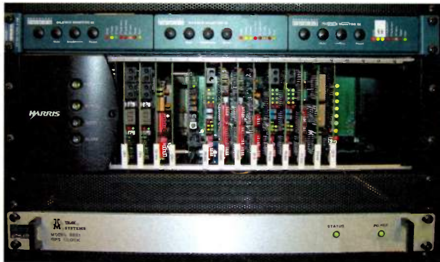
An installed Harris Intraplex SynchroCast quietly coordinates transmission.
