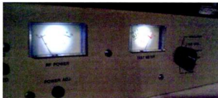
Fig. 1: Replace incandescent bulbs with LEDs to illuminate the meters. Bonus: The glow serves as a power 'on' indicator.
