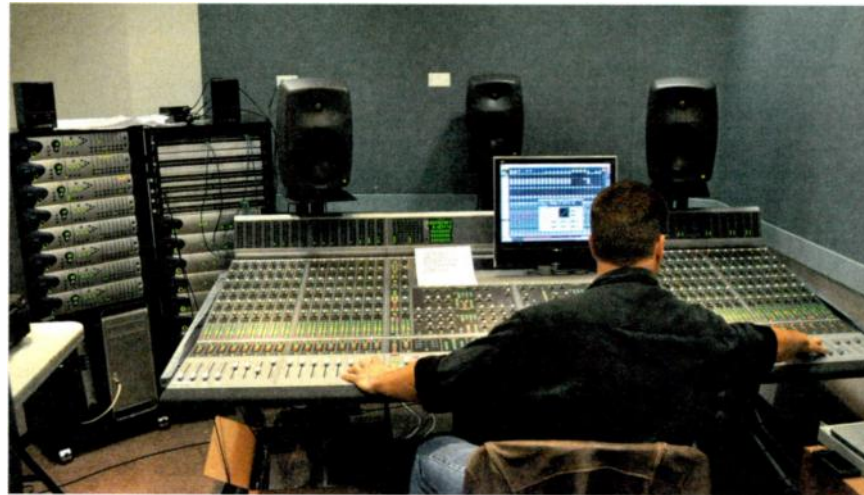
Control Room for the P.C. Richard & Son Theater
