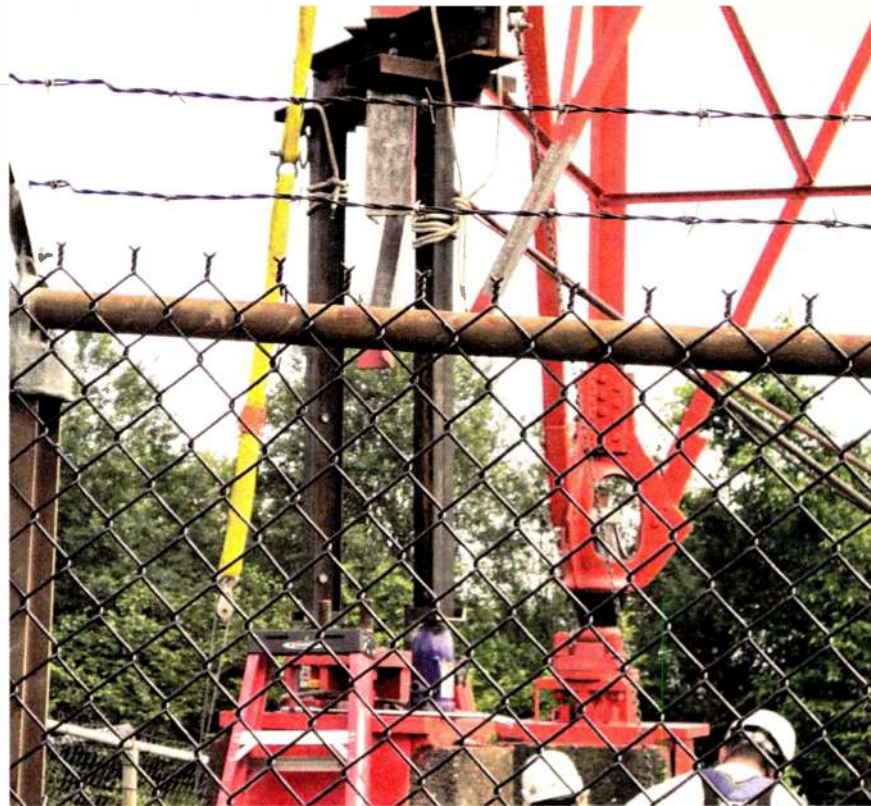
The lifting bracket is visible with the insulator assembly out.
