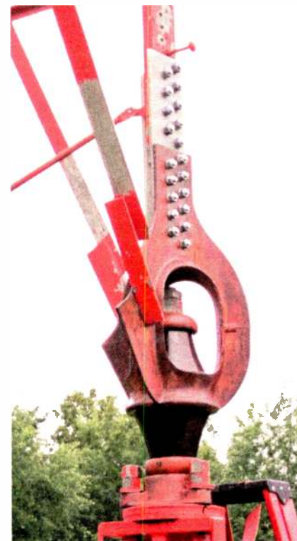
One of the completed insulator replacements, ready for priming and painting ... without the overspray! Note the bare metal adapter plate bolted to the tower leg.
