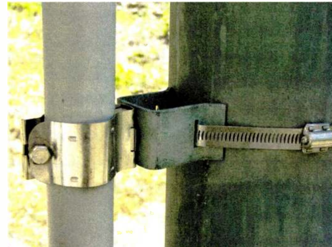
Fig. 5: Secure conduit is less of a temptation to vandals.
