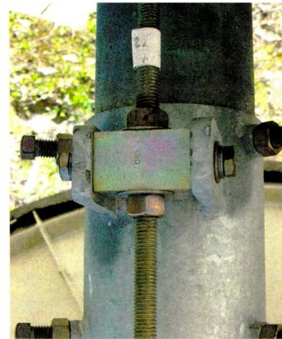
Fig. 4: Wrapping electrical tape around the threads will work, but it can be easily removed.
