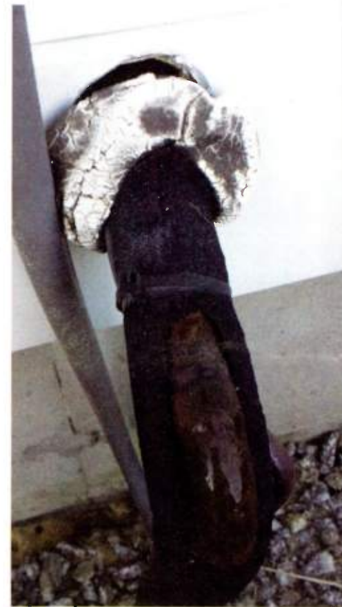
Fig. 2: Inspect sealed entries for shrinkage, which opens the door to pests.
