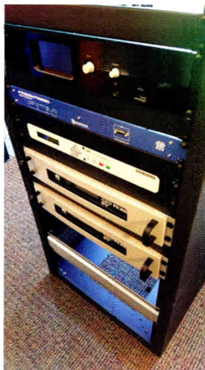
Fig. 1: Why not build that translator rack in your shop rather than on site?
