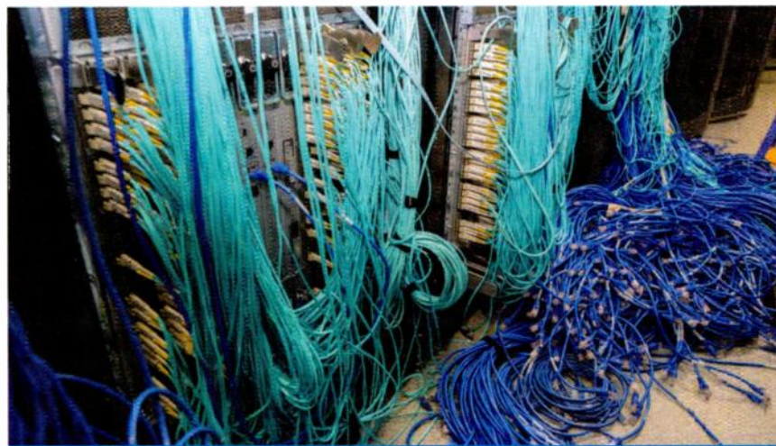
An example of the thousands of cables that need to be managed when moving servers to a commercial service provider.
