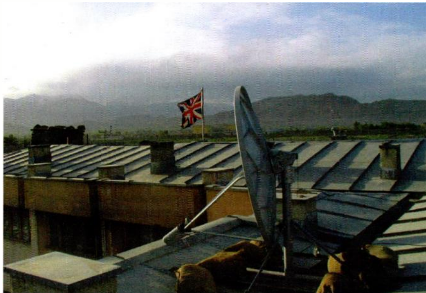
A view from an installation in Kabul in 2002. "At a look angle of 18 degrees, getting line of site to the satellite often meant mounting dishes at height and often on a roof," Ramsay said. "Also it meant our offset dishes looked as though they were pointing down, which confused people."
