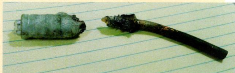
Fig. 6: A broken crimp/pin connecting one of the service drop cables on a pole pig transformer
