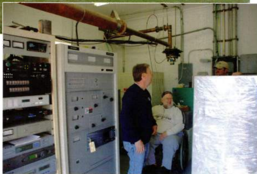
News Director John Daniel, Chief Engineer Michael Holderfield and "Love Zone" host and sales rep Brad Bailey inspect a new transmitter.
